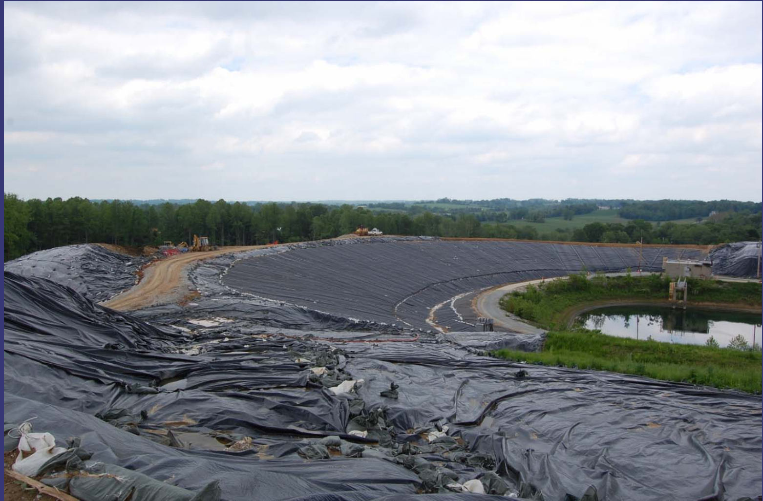
Mix of completed, partially complete, and temporary liners around the stormwater pond.
