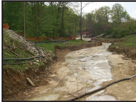
View looking west of Bailey Scales Road - post excavation but prior to restoration
