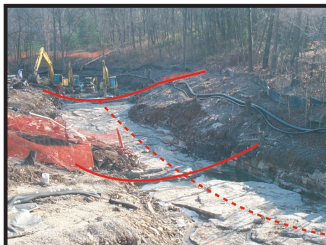
Trench excavation in bedrock as part of the Site Source Control activities near GMs historic outfall
