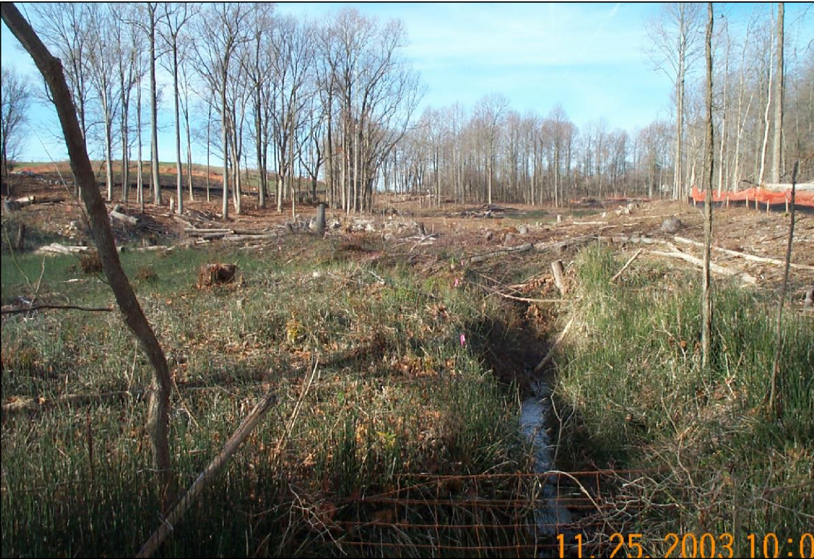
PHOTO No.78, N AOI 4: LOOKING WEST ALONG CREEK ALIGNMENT PRIOR TO EXCAVATION (NOV. 2003)
