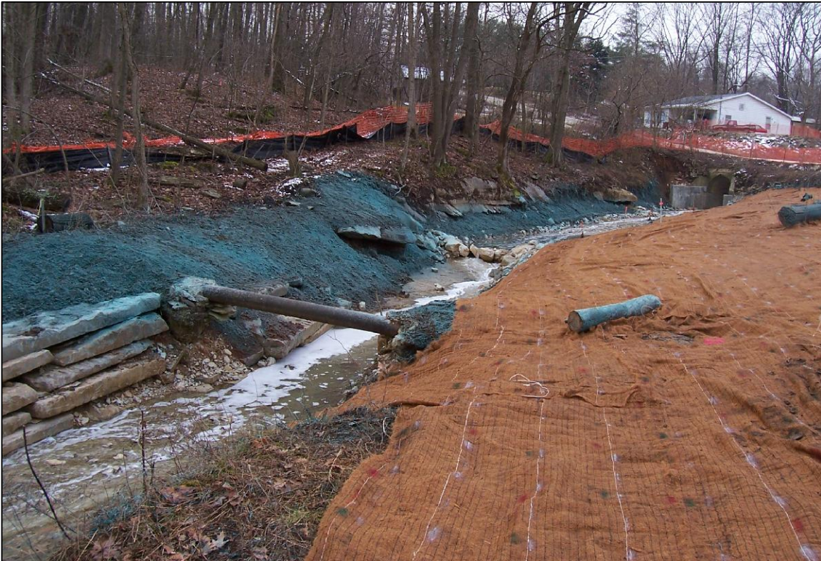
PHOTO No.34, PARCEL 5 & 8: INSTALLATION OF EROSION CONTROL MATS ALONG PARCELS 5 AND 8 (FEB. 2005)
