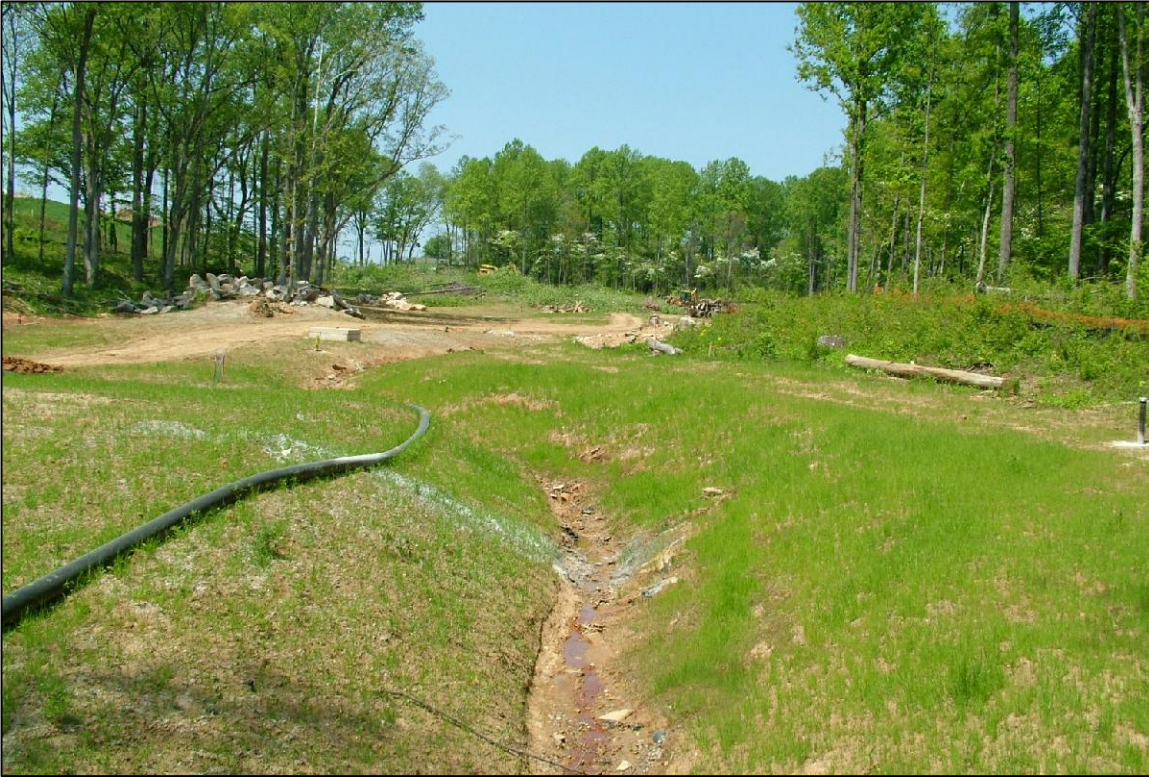
PHOTO No.83, N AOI 4: RESTORATION PROGRESS LOOKING WEST TOWARDS AOI 4 ALONG CREEK CHANNEL (NOV. 2003)
