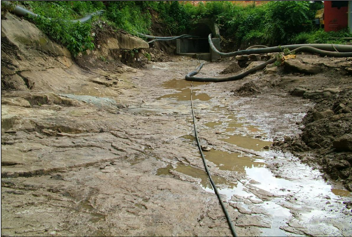
PHOTO No.33, PARCELS 5 & 8: FACING UPSTREAM (SOUTHWEST) TOWARDS CULVERT AT BAILEY SCALES ROAD ALONG EXCAVATED AND CLEANED CREEK ALIGNMENT (JUL. 2004)
