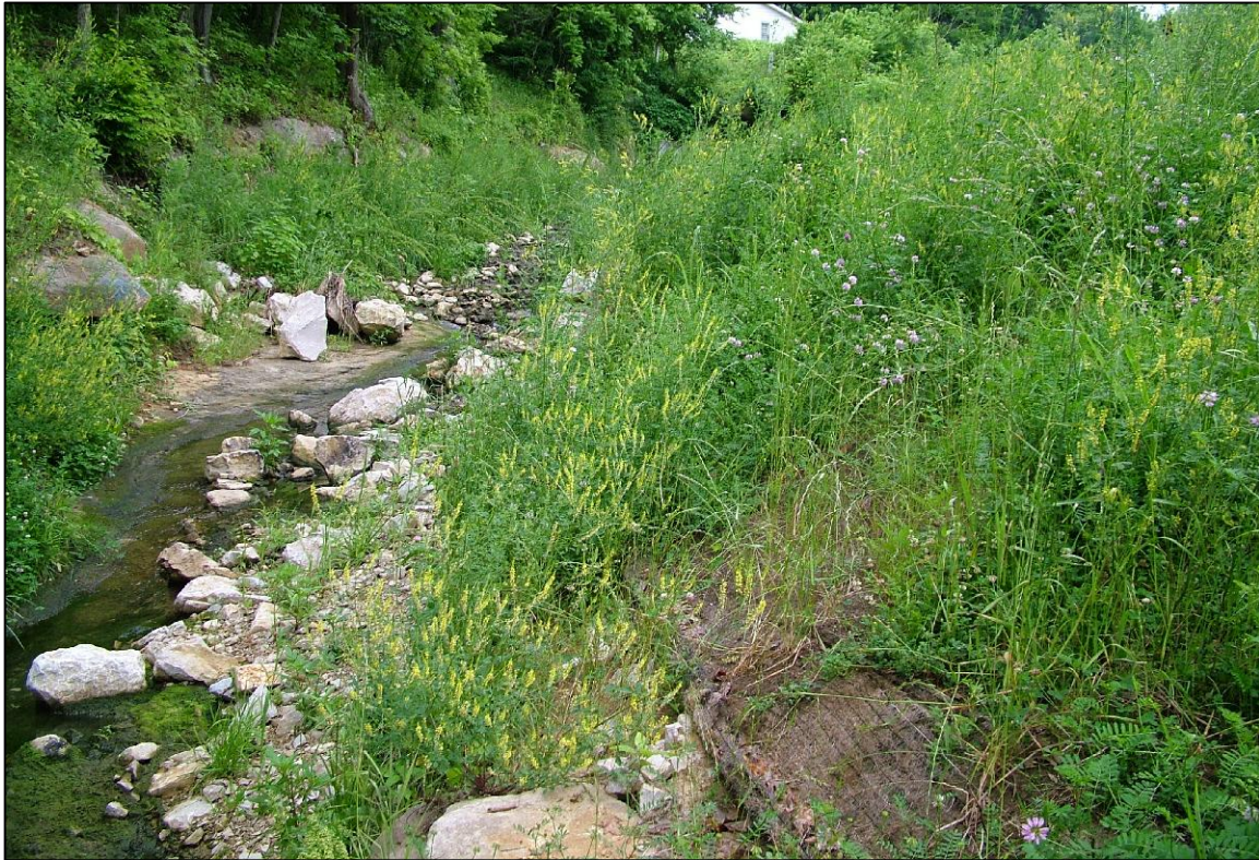
PHOTO No.35, PARCELS 5 & 8: RESTORED WALL ON PARCEL 5 AT BAILEY SCALES CULVERT (JUN. 2006)
