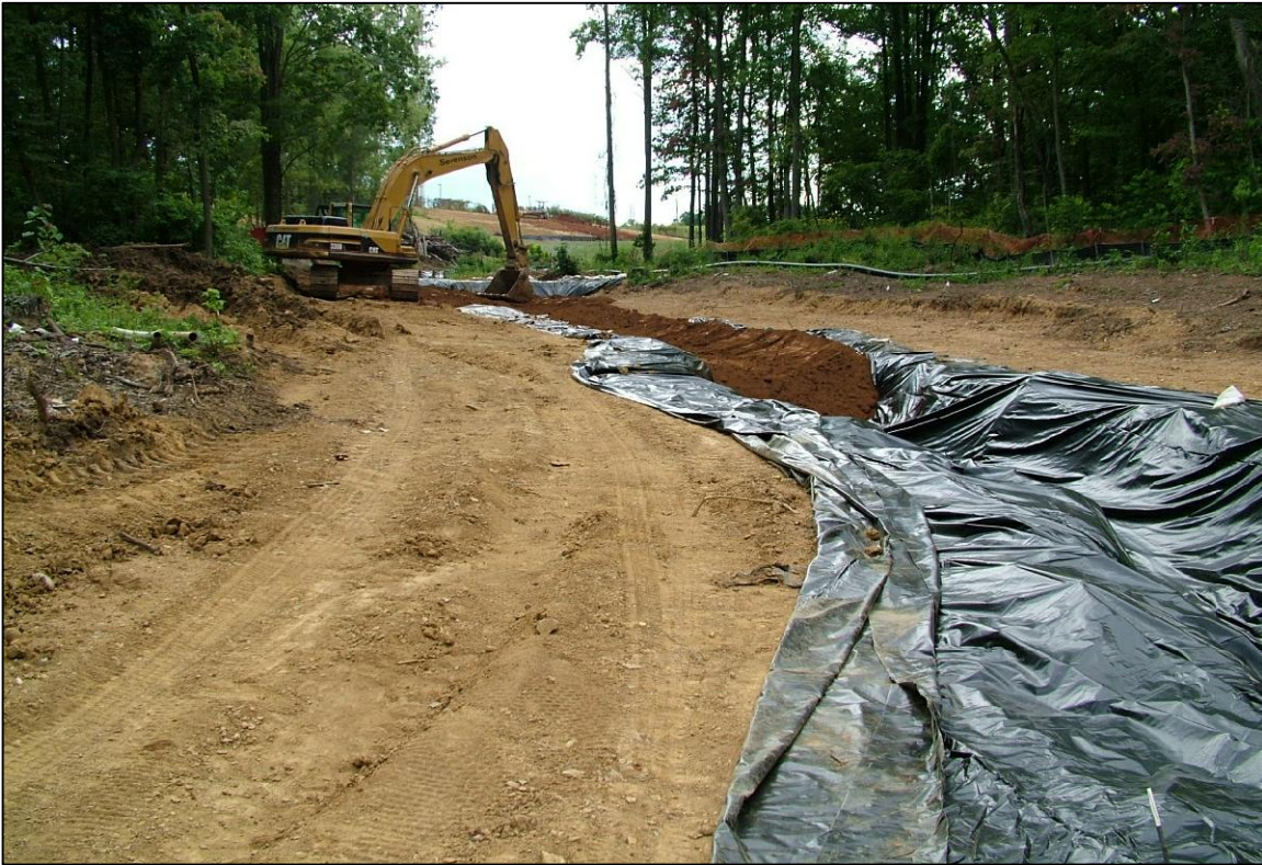
PHOTO No.82, N AOI 4: BACKFILLING EXCAVATION SEPARATING BEDROCK FROM CHANNEL WITH LINER (AUG. 2004)
