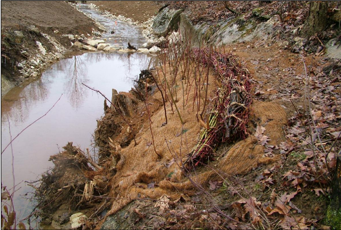
PHOTO No.46, PARCELS 8 & 10: RESTORED CREEK FACING DOWNSTREAM; FASCINE BUNDLE IN THE FOREGROUND (FEB. 2005)
