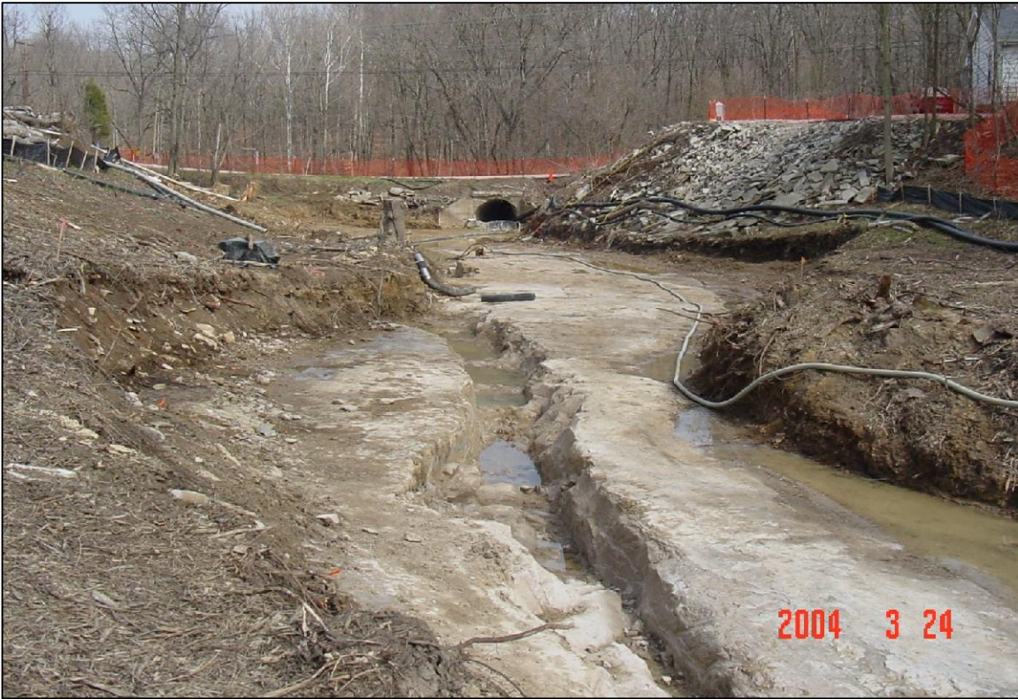
PHOTO No.24, PARCEL 5: BROKEN OUT FRACTURE LOOKING DOWNSTREAM ALONG PARCEL 5 & 6 ALIGNMENT (MAR. 2004)
