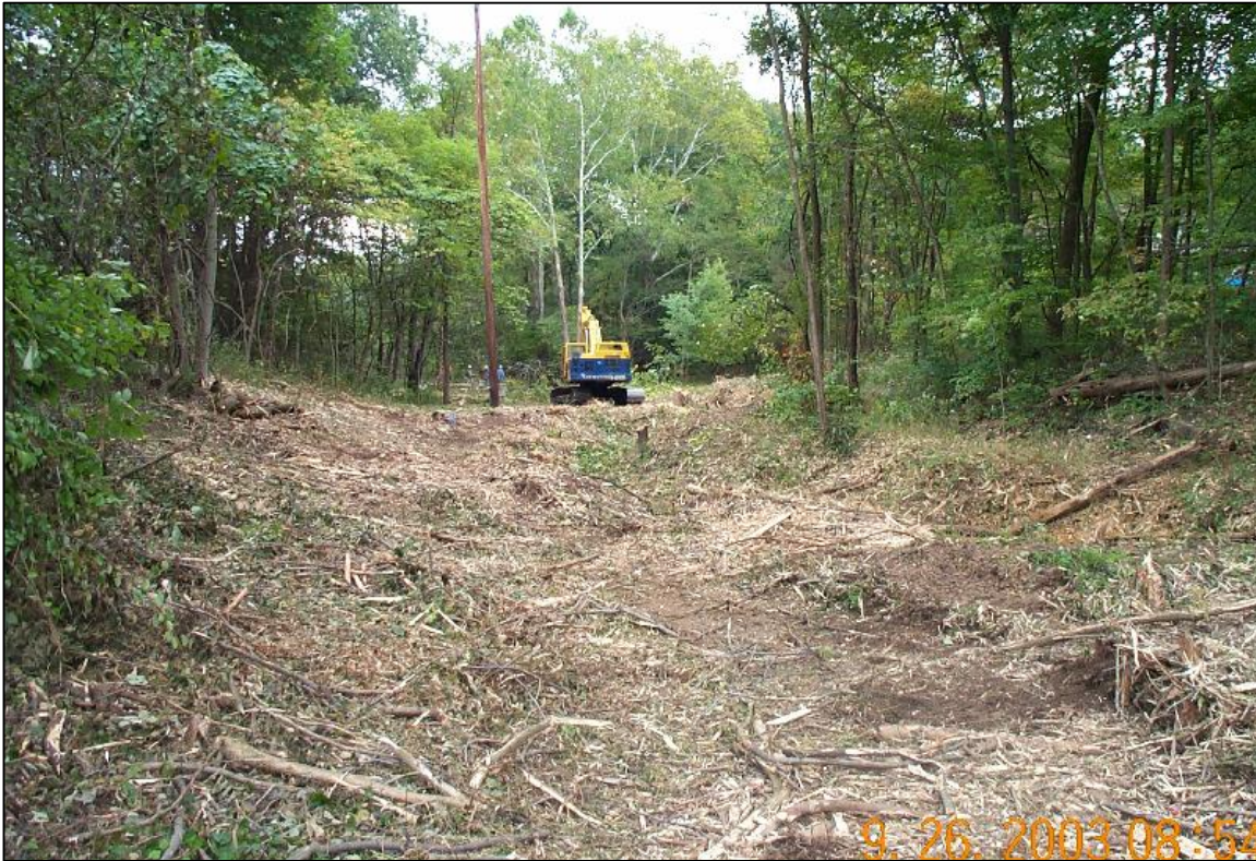
PHOTO No.14, PARCEL 4: MOBILIZATION ON PARCEL 4, FACING DOWNSTREAM (EAST) ALONG CLEARED CREEK ALIGNMENT (SEP. 2003)
