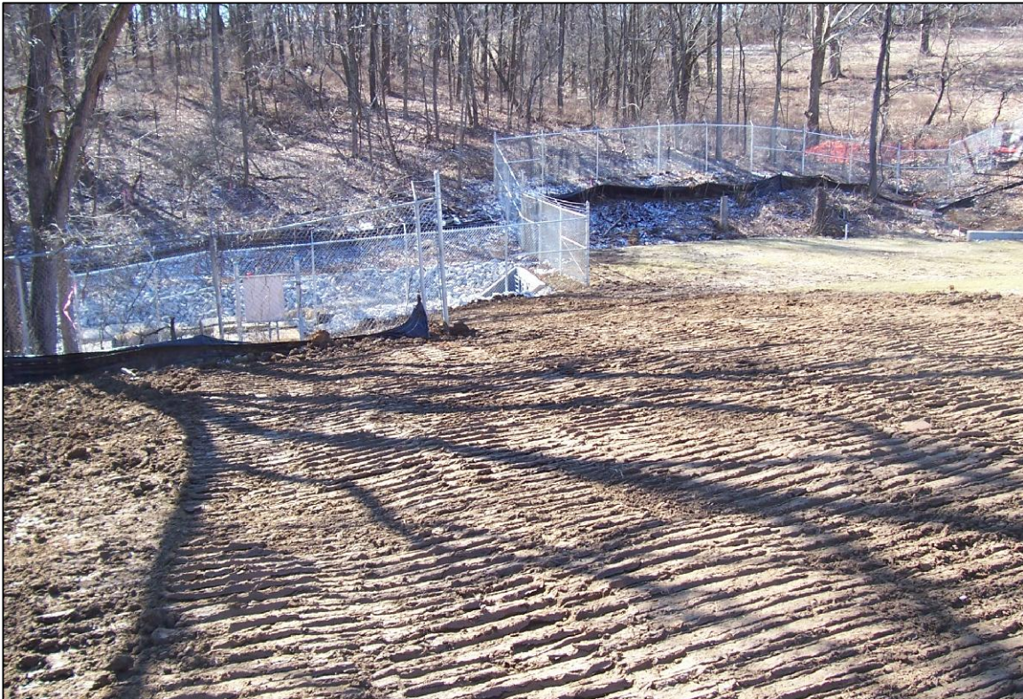
PHOTO No.12, PARCEL 205: POST-BACKFILLING ON PARCEL 205 FACING SOUTH LOOKING TOWARD PARCEL 3 AND 4 (MAR. 2005)
