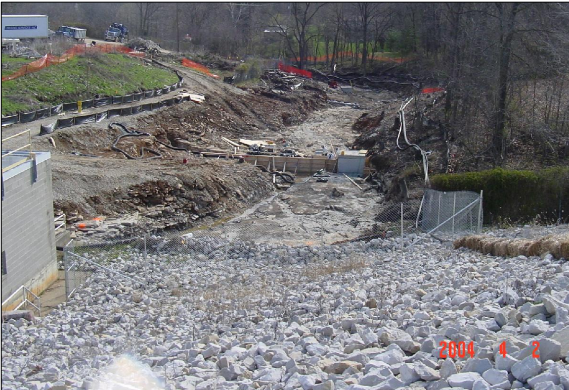
PHOTO No.6, PARCEL 3: CLEANED EXCAVATION AND INSTALLATION OF SOME SITE SOURCE CONTROL FEATURES FACING DOWNSTREAM (EAST) (APR. 2004)
