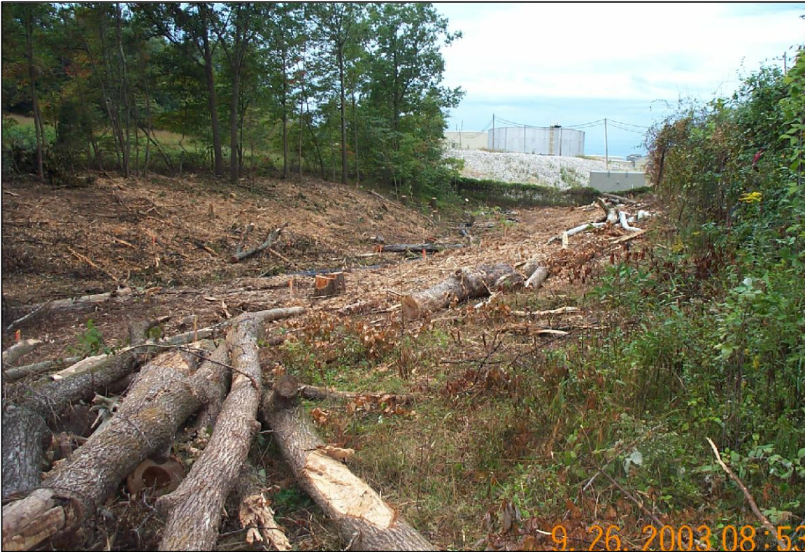
PHOTO No.2, PARCEL 3: MOBILIZATION ON PARCEL 3 CREEK ALIGNMENT, FACING UPSTREAM (WEST) (SEP. 2003)
