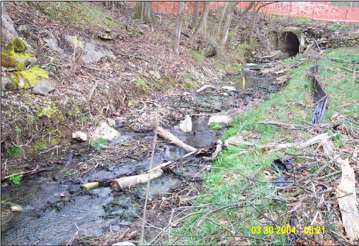
PHOTO No.32, PARCELS 5 & 8: MOBILIZATION ALONG PARCEL 5 AND 8 FACING UPSTREAM (SOUTHWEST) TOWARDS BAILEY SCALES ROAD (MAR. 2004)
