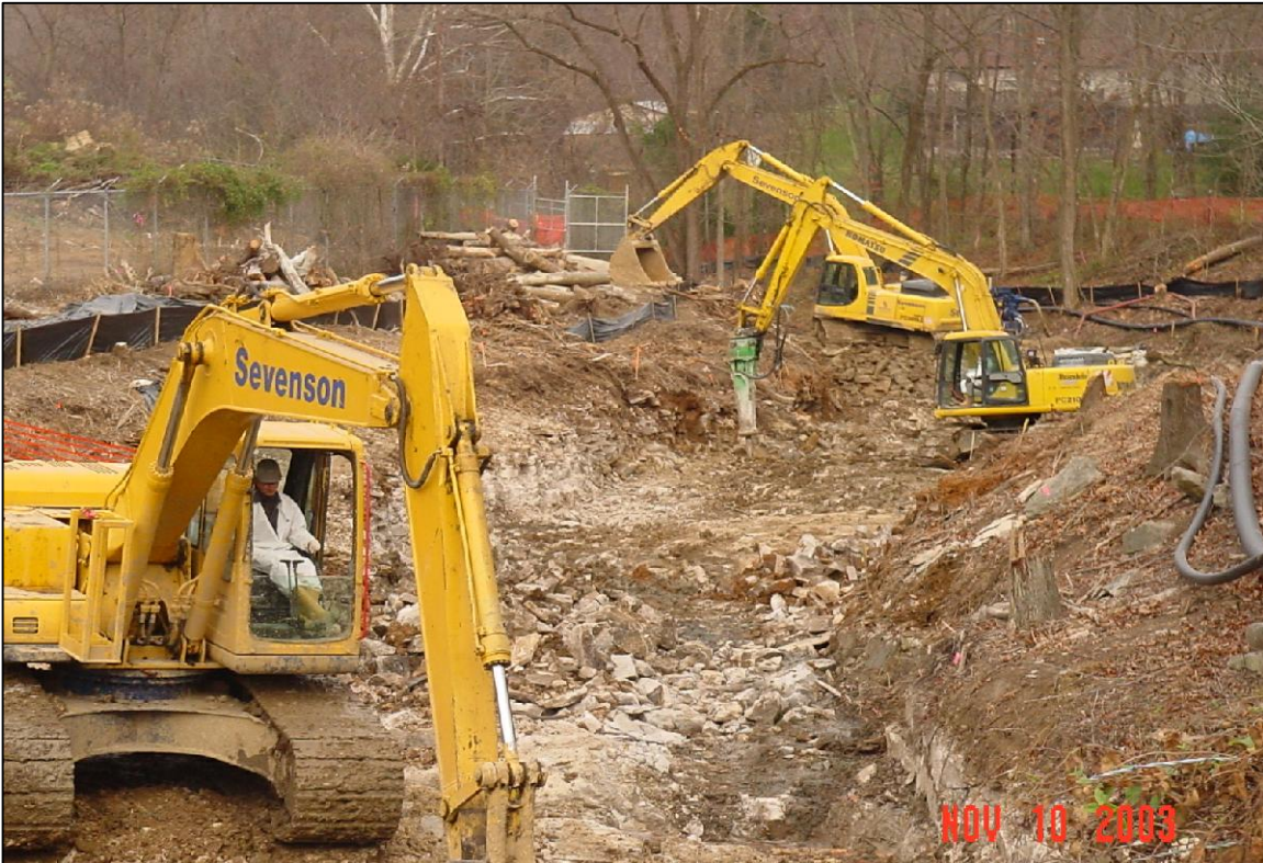
PHOTO No.4, PARCEL 3: ROCK BREAKING ALONG CREEK ALIGNMENT FACING DOWNSTREAM (EAST) (NOV. 2003)
