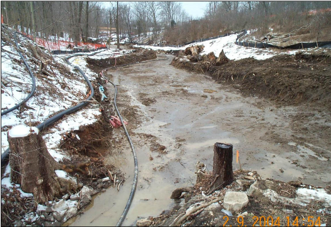
PHOTO No.23, PARCEL 5: EXCAVATED CREEK CHANNEL FACING UPSTREAM (WEST) ALONG CREEK ALIGNMENT (FEB. 2004)
