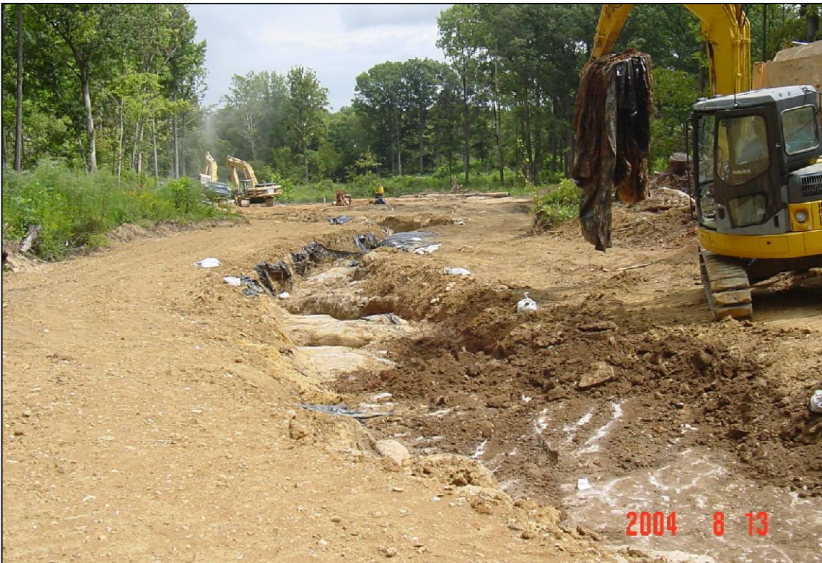
PHOTO No.80, N AOI 4: EXCAVATION PROGRESS LOOKING EAST ALONG CREEK ALIGNMENT (AUG. 2004)
