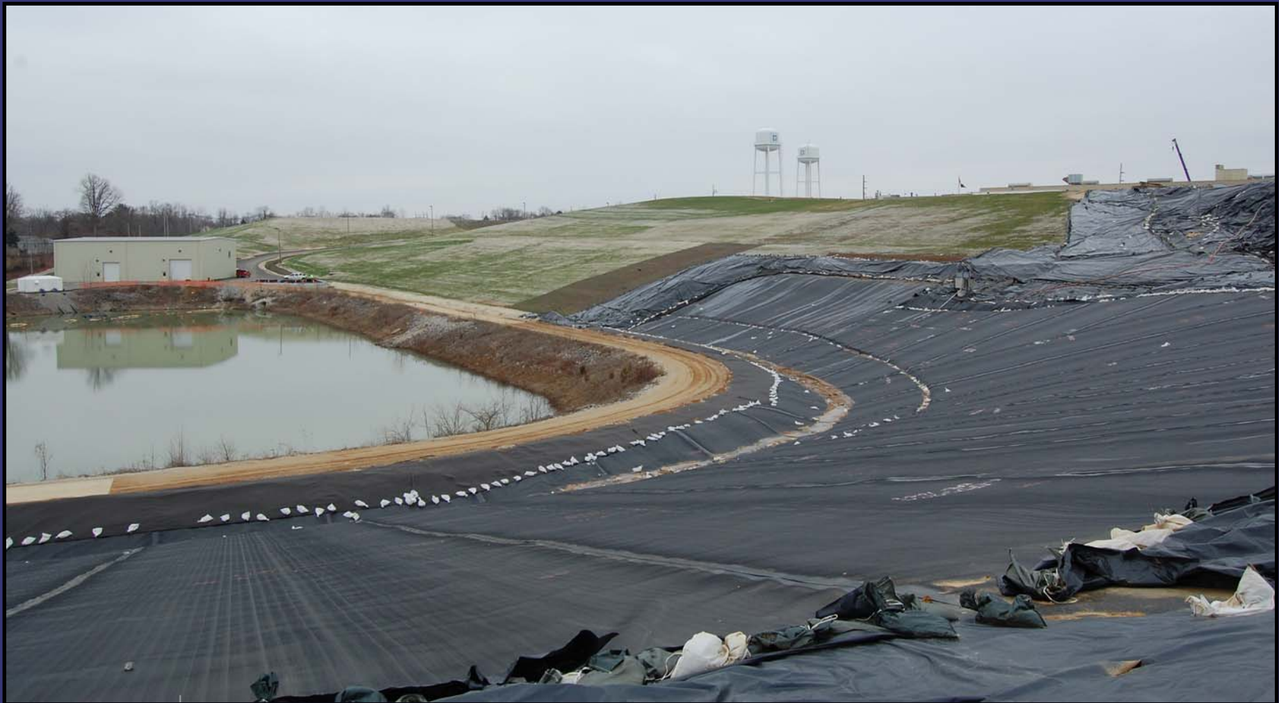
Mix of completed, partially complete, and temporary liners around the stormwater pond.
