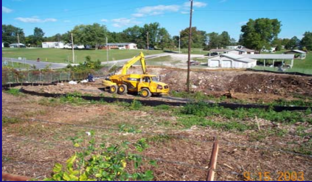
Looking north towards excavation area (northern tributary) – north of AOI 4 and south side of Parcel 401
