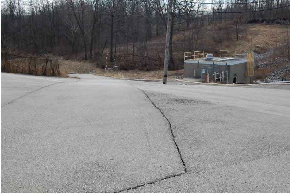
Photo 26: EA2 facing east, cracks in asphalt west of Parcel 205
