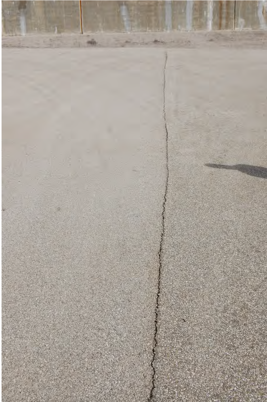
Photo 25: EA2 crack near WWTP aeration basin facing north
