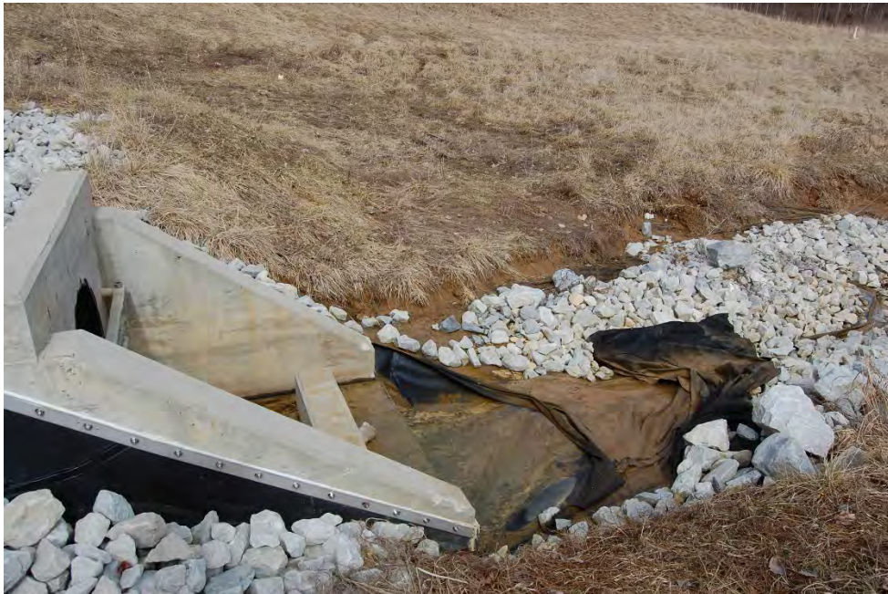
Photo 22: EV9 rip rap erosion at storm drain into detention basin #2 facing north
