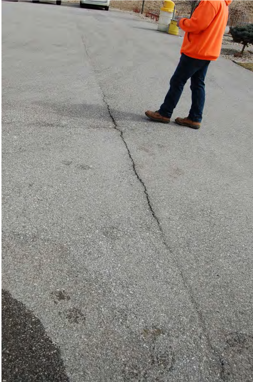
Photo 30: WA surficial asphalt crack facing east
