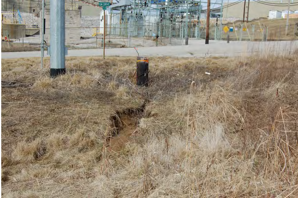
Photo 9: EV6 erosion rut outside cap limit
