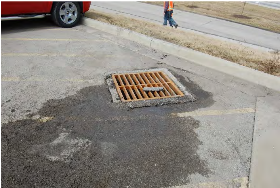
Photo 32: WA damaged asphalt surface near catch basin
