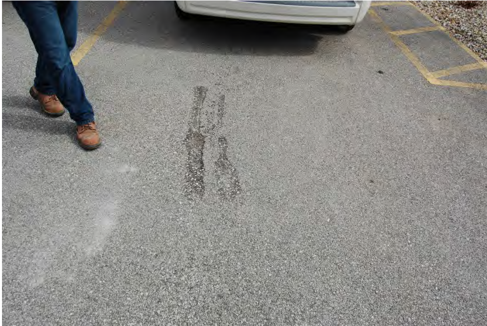
Photo 31: WA asphalt gouge in parking spot
