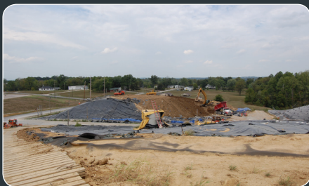
EAST PLANT AREA RECEIVING GRADING MATERIAL FROM STOCKPILE WEST OF PEERLESS ROAD.
