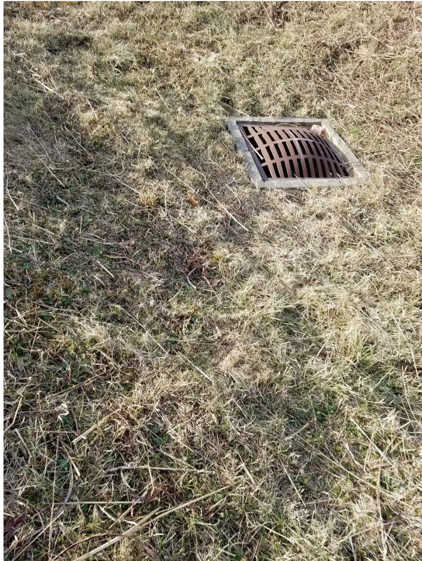
Photo 19: EV9 East Plant Area Cover surface water drainage.
