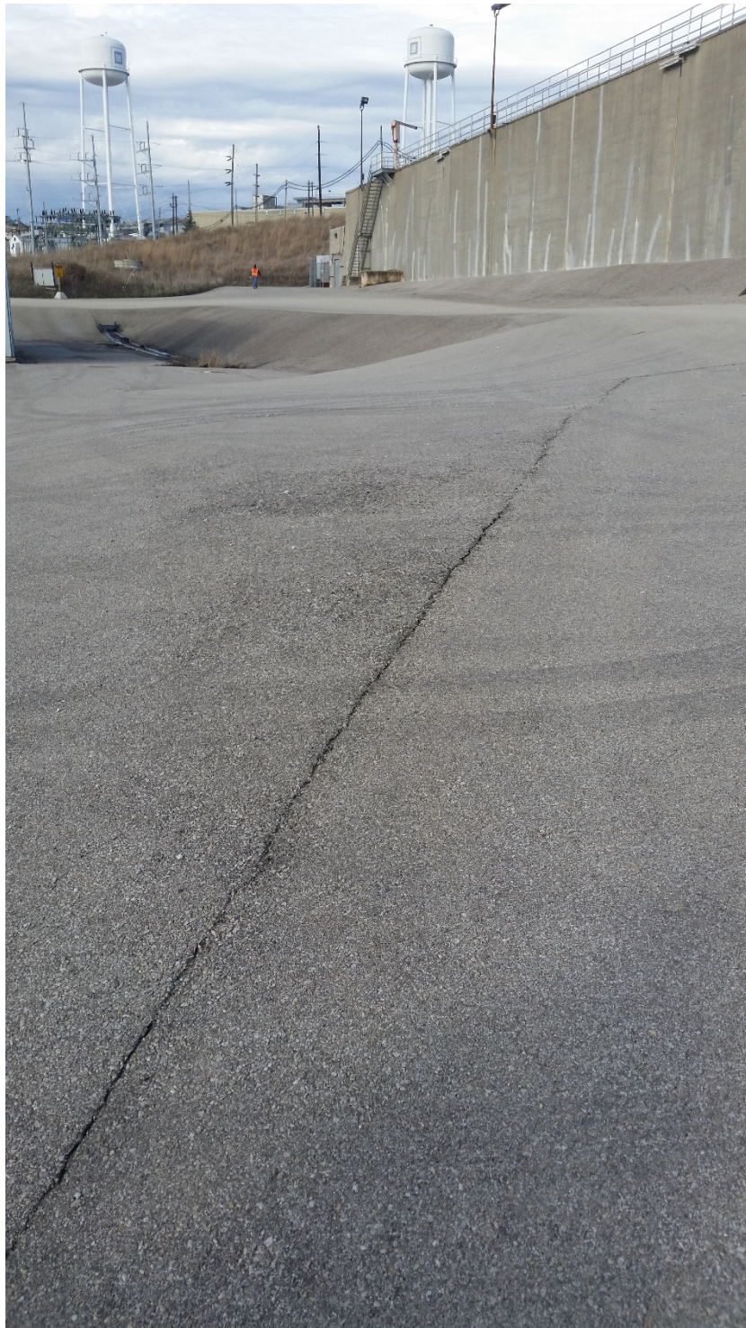
Photo 35: EA2 facing west, cracks in asphalt west of Parcel 205.
