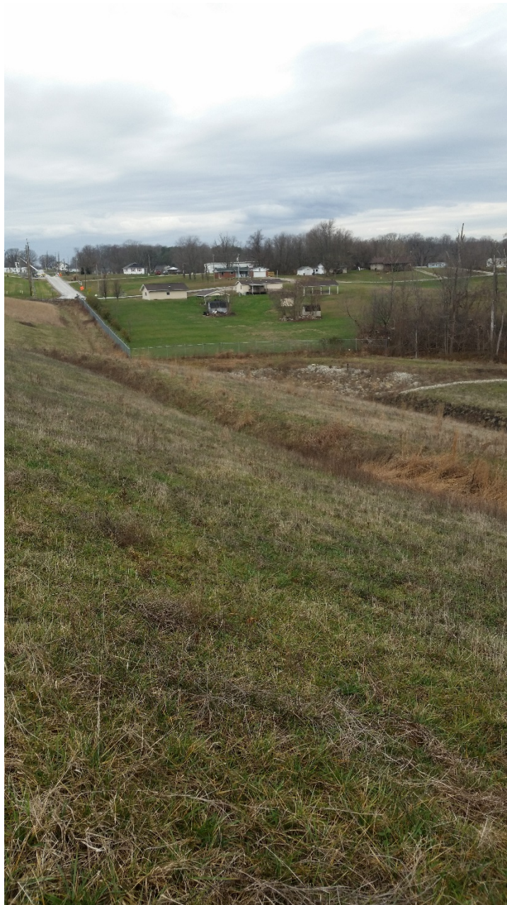
Photo 23: ES5 drainage swale facing west.
