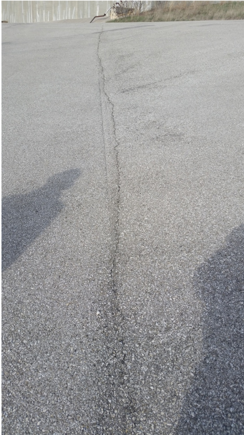
Photo 34: EA2 facing north, cracks in asphalt west of Parcel 205.
