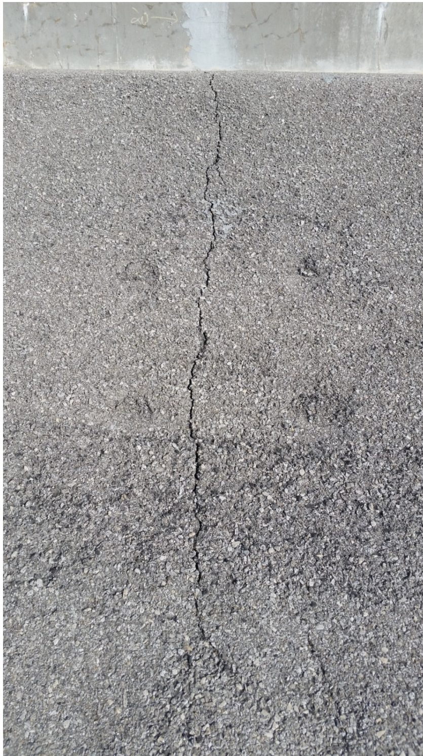
Photo 33: EA2 crack near WWTP aeration basin facing north.
