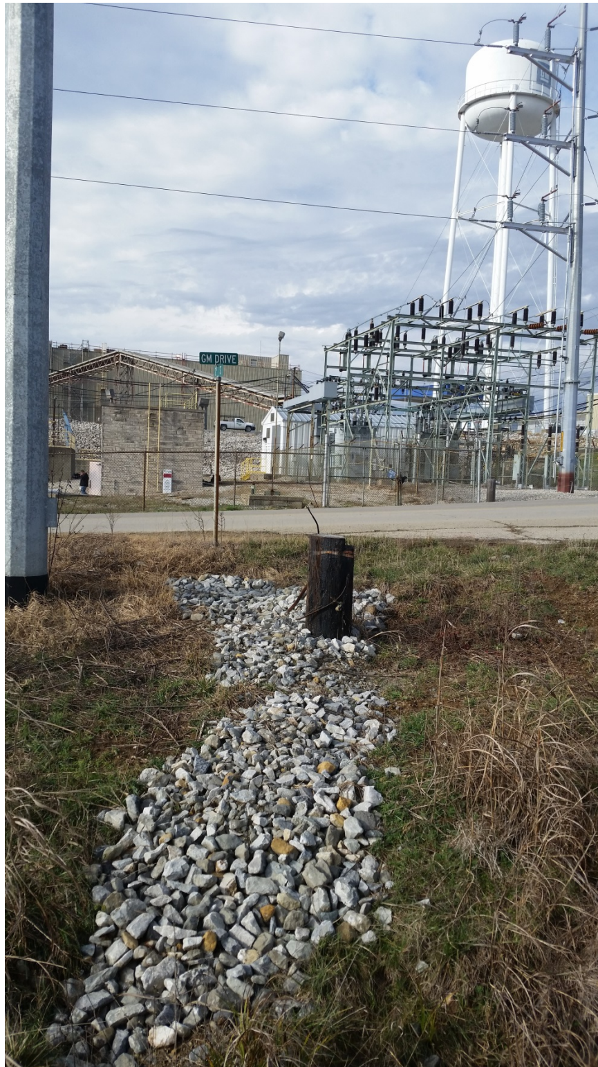
Photo 10: EV6 erosion rut repairs outside cap limit.
