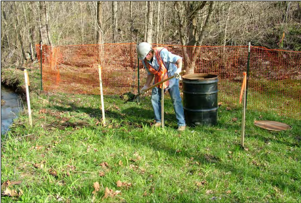
PHOTO 19: PARCEL 57 - HAND EXCAVATION OF TOP 4 TO 6 INCHES OF SOIL (FACING WEST). APRIL 2006
