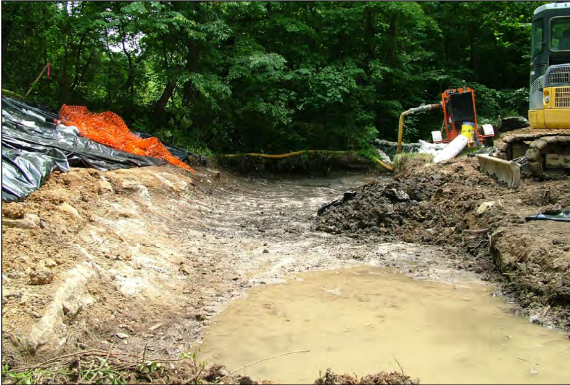
PHOTO 29: PARCEL 60 - LOOKING ALONG THE CREEK AT EXCAVATION TO BEDROCK (FACING EAST). JULY 2006
