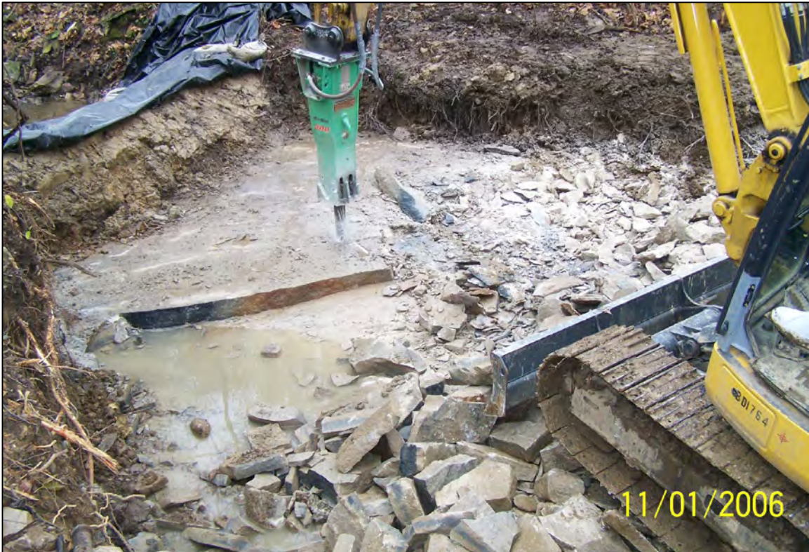
PHOTO 34: PARCEL 60 & 61 - BREAKING OUT ROCK IN THE CREEK WITH A HYDRAULIC RAM (FACING SOUTH). NOVEMBER 2006
