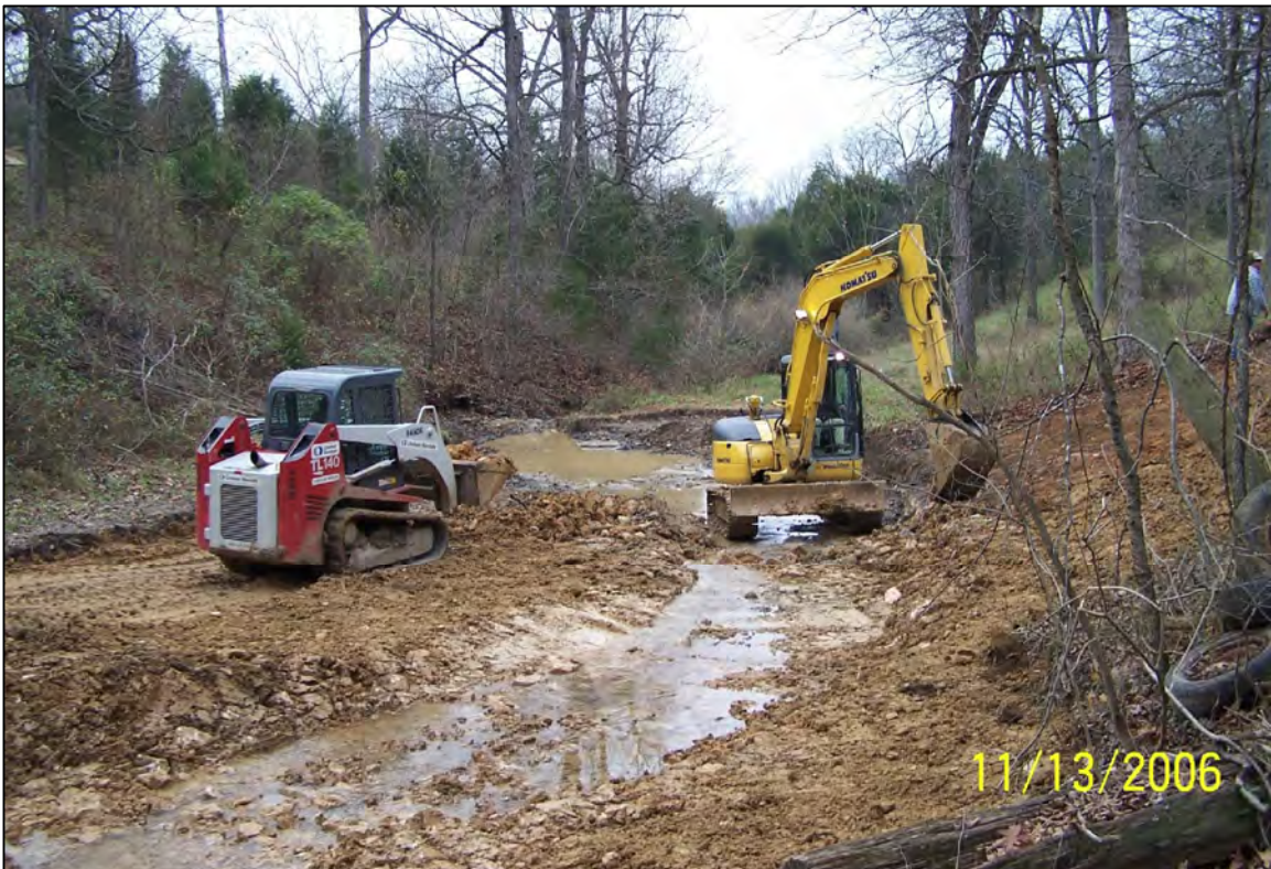
PHOTO 36: PARCEL 60 - BACKFILLING CREEK WITH IMPORTED FILL MATERIAL FOR RESTORATION (FACING WEST). NOVEMBER 2006
