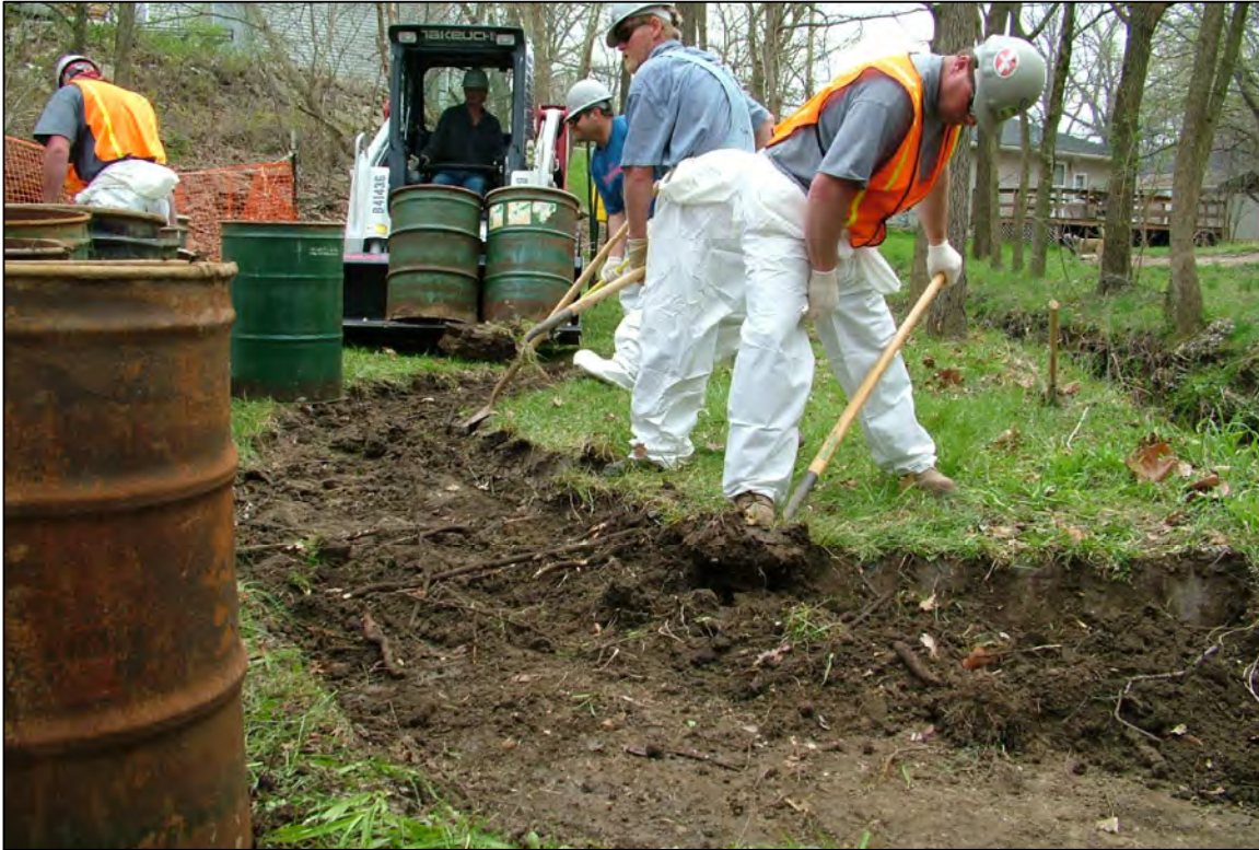
PHOTO 21: PARCEL 57 - HAND EXCAVATION AND PLACEMENT INTO DRUMS FOR SOIL REMOVAL (FACING EAST). APRIL 2006
