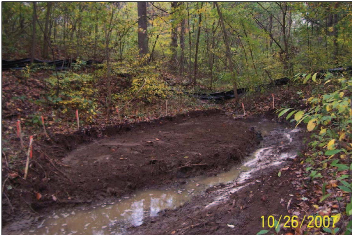
PHOTO 04: PARCEL 387/389 - SILTATION FENCES TO PREVENT EROSION AND MIGRATION OF DEBRIS FROM THE WORK AREA (FACING NORTH). OCT-07
