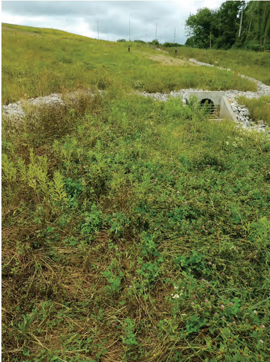
Photo 9: ES9 East Plant Area Cover detention basin 2 inlet
