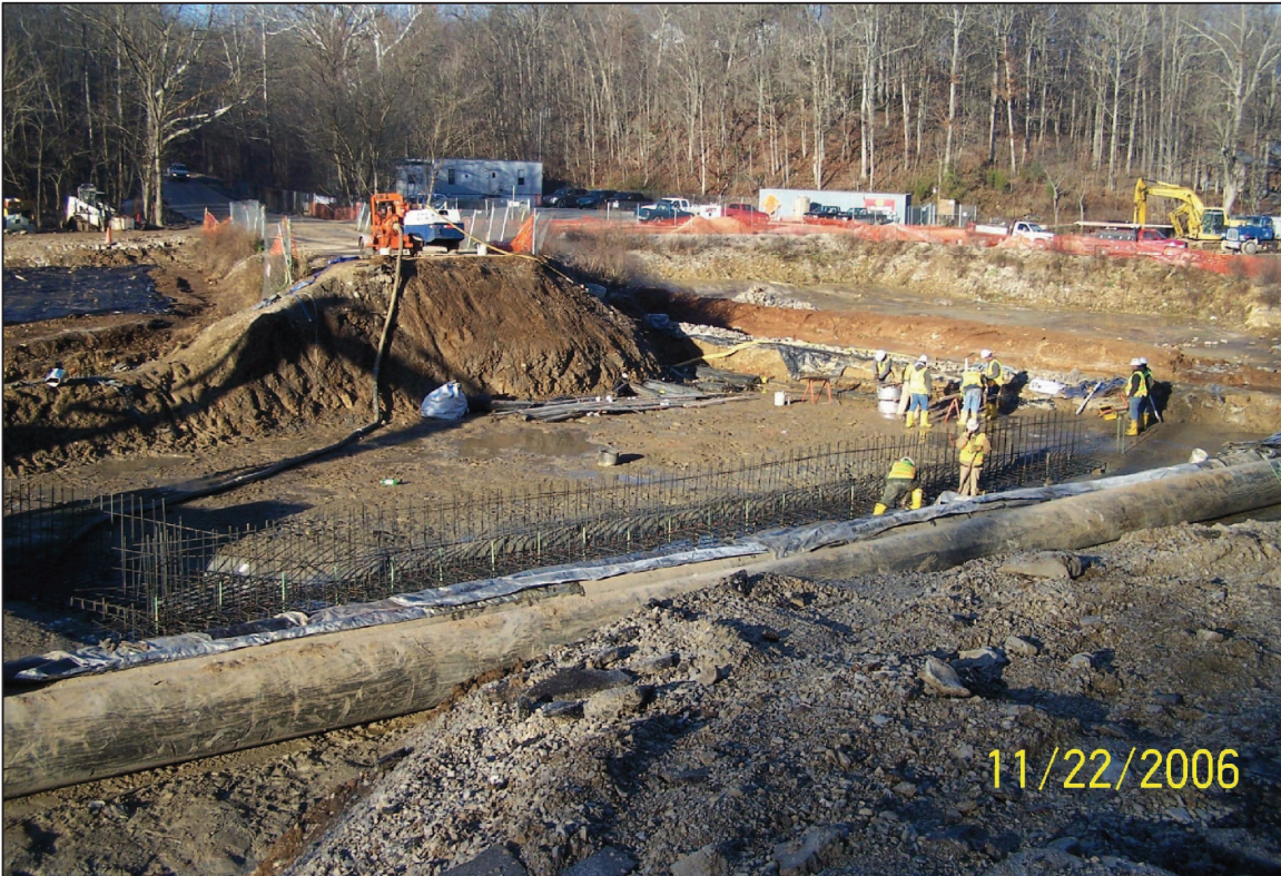
PHOTO No. 22, PARCEL 22: VIEW OF THE REMOVED SECTION OF ROAD AND PREPARATION OF STEM WALLS. (NOV. 2006)
