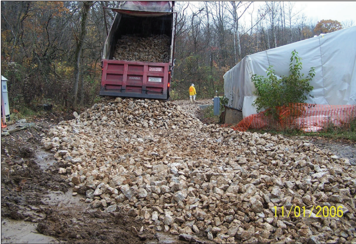
PHOTO No. 21, PARCEL 22: CREATION OF THE TEMPORARY ACCESS ROAD FOR RESTORATION CONSTRUCTION. THE STONE WAS EVENTUALLY INCORPORATED INTO THE CREEK SUBSTRATE. (NOV. 2006)
