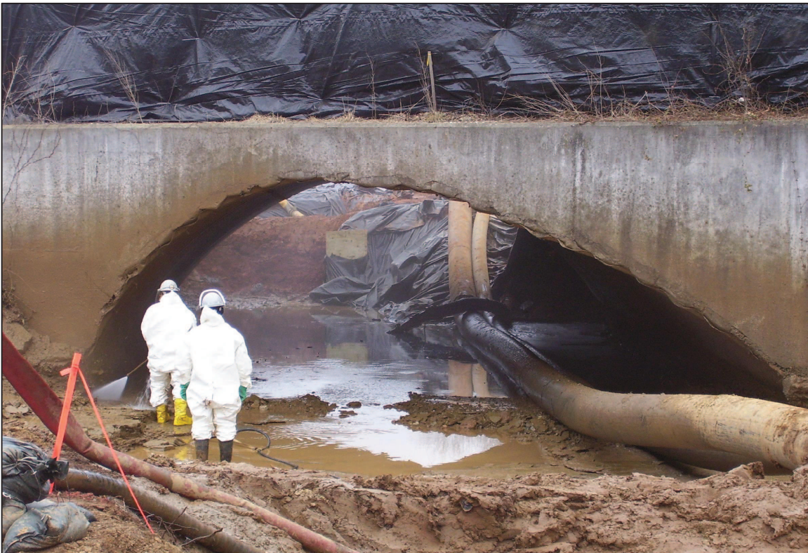
PHOTO No. 14, PARCEL 22: POWERWASHING UNDER THE BROOMSAGE ROAD CULVERT TO PREPARE FOR DAM CONSTRUCTION. (MAR. 2006)
