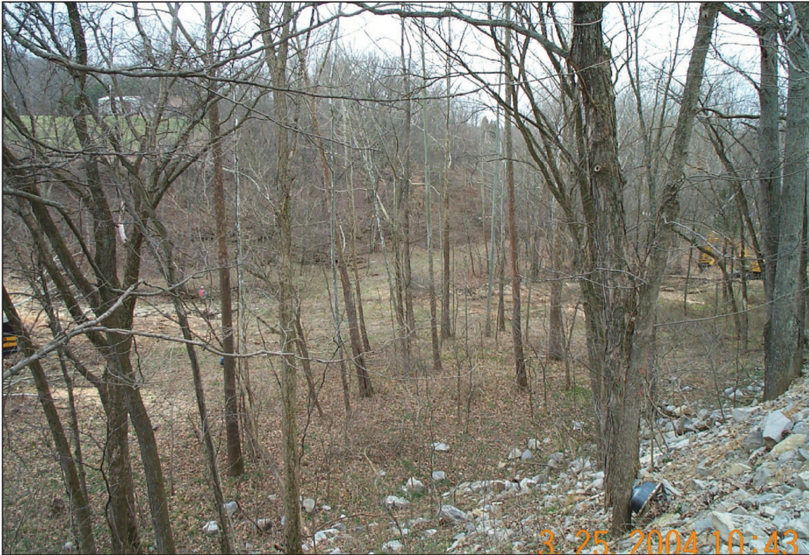
PHOTO No. 4, PARCEL 22: TREE CLEARING ACTIVITIES LOOKING DOWN INTO THE FLOODPLAIN FROM BROOMSAGE ROAD. (MAR. 2004)
