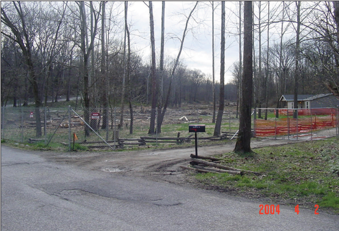
PHOTO No. 5, PARCEL 22: TREE CLEARING OF THE PARCEL PRIOR TO EXCAVATION. (APR. 2004)
