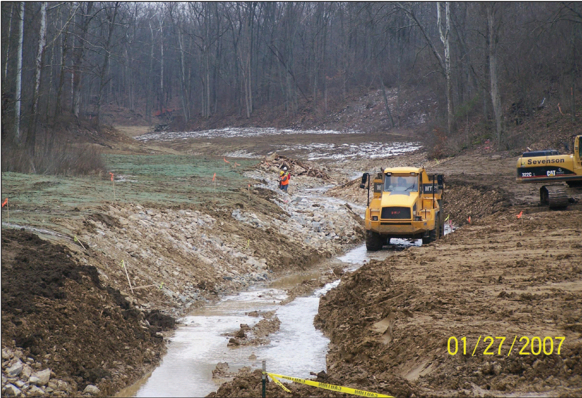
PHOTO No. 26, PARCEL 22: BACKFILLING AND GRADING OF MATERIAL WITHIN THE CREEK. (JAN. 2007)
