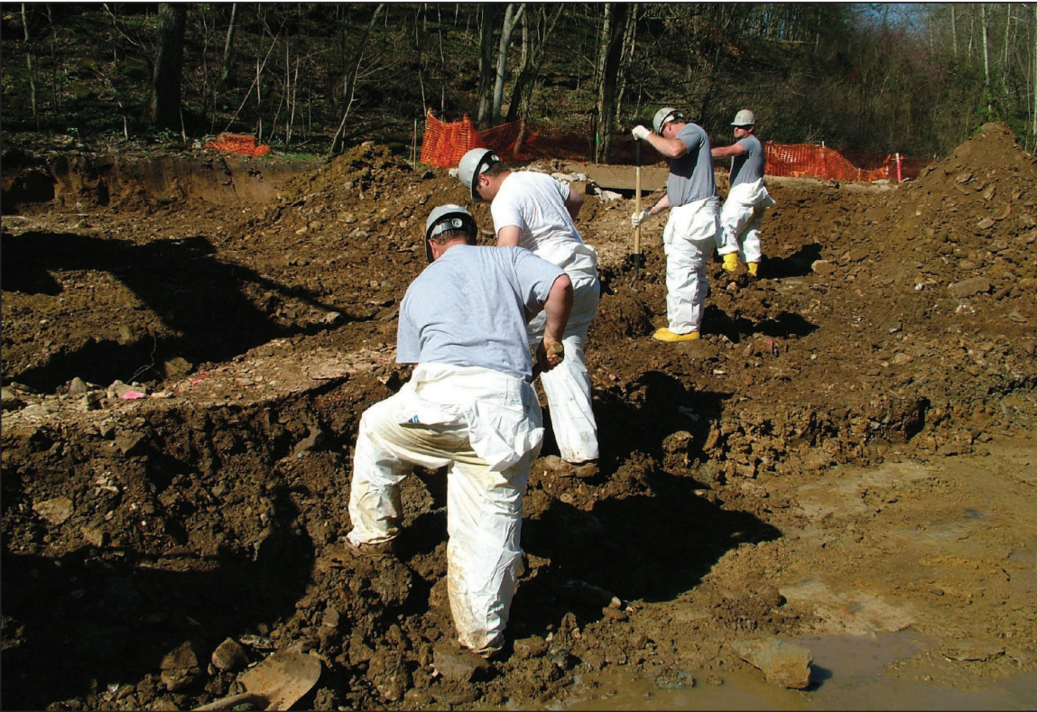
PHOTO No. 16, PARCEL 22: HAND DIGGING ADDITIONAL MATERIAL NEAR A GAS LINE ON THE PROPERTY. (APR. 2006)
