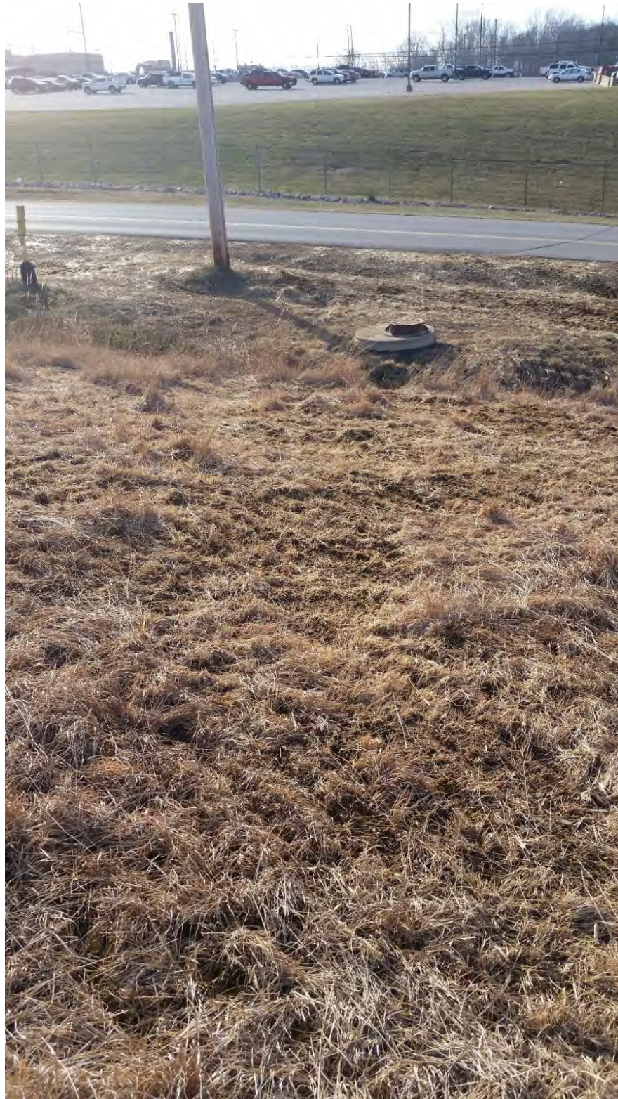
Photo 5: Vegetative growth along GM Drive, west of ES3 East Plant Area Cover facing west
