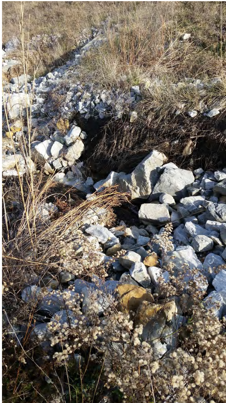
Photo 7: Rip-rap erosion at ES6 East Plant Area Cover
