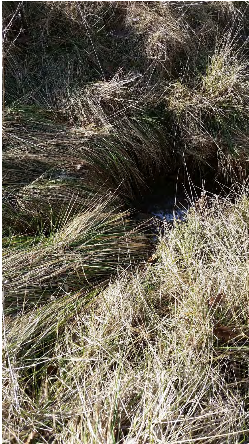
Photo 15: Former animal burrow near ES6 East Plant Area Cover
