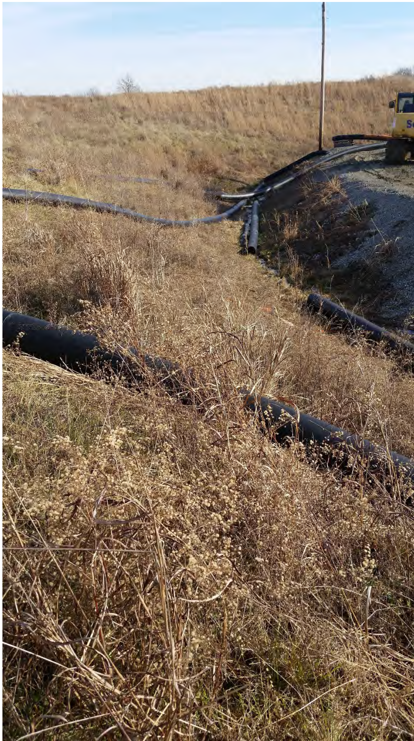
Photo 9: Temporary pumping lines in ES1 East Plant Area Cover at north end of Pond
