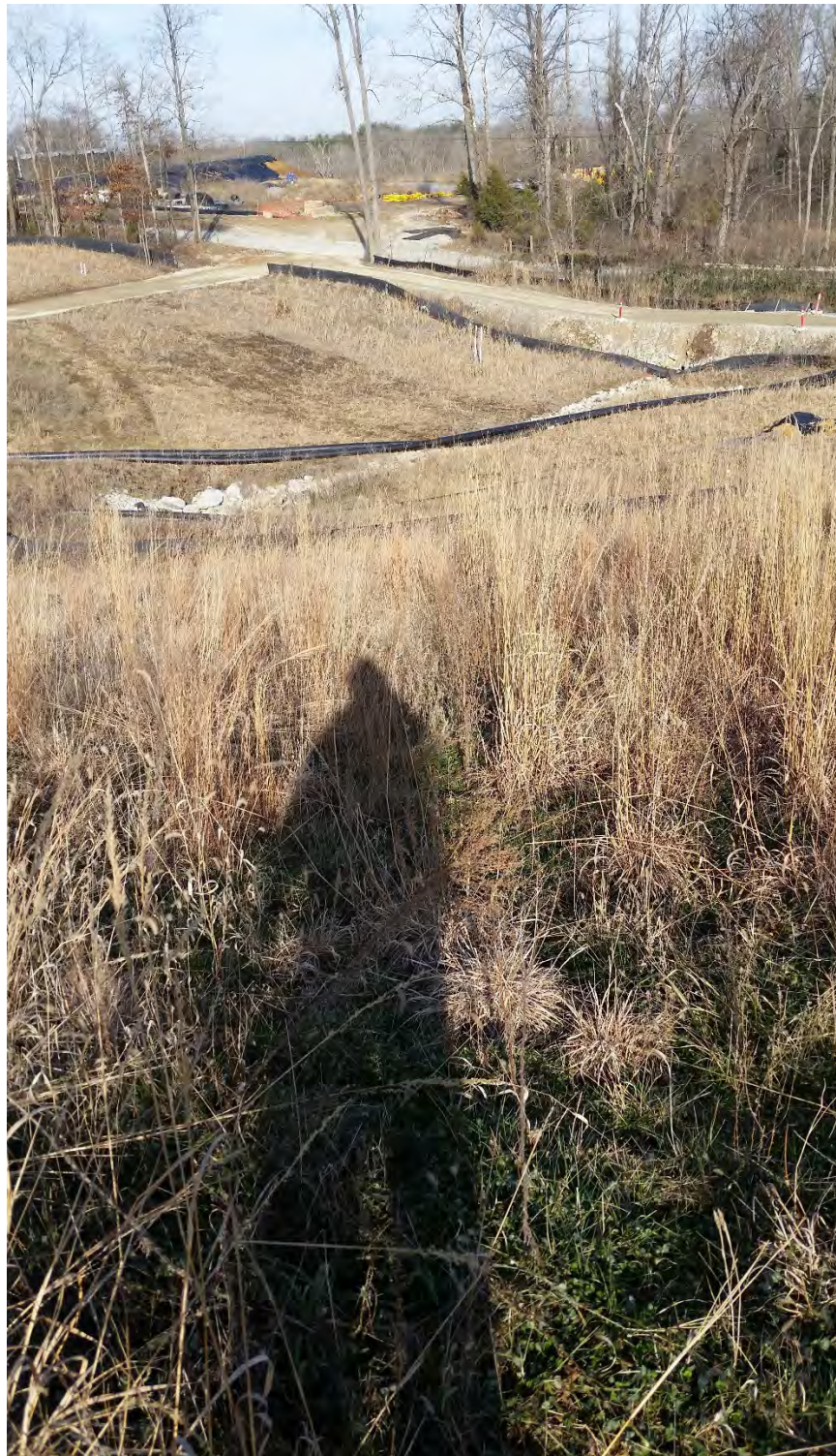
Photo 12: EV4 East Plant Area Cover looking northeast toward ES11 East Plant Area Cover
