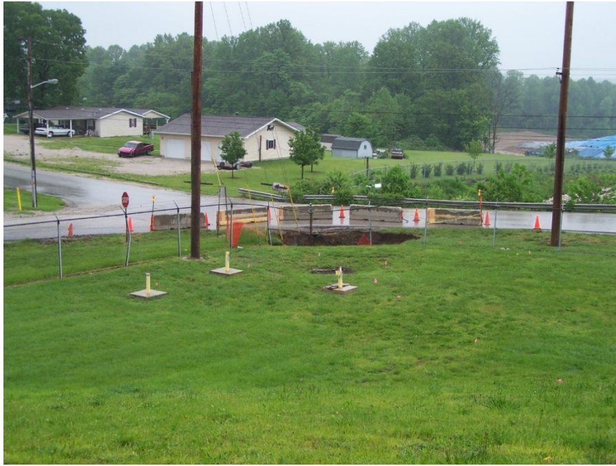
Photo No. 1: MH-ST-43 - Pre-construction conditions (showing sinkhole), facing northeast. April 2008.
