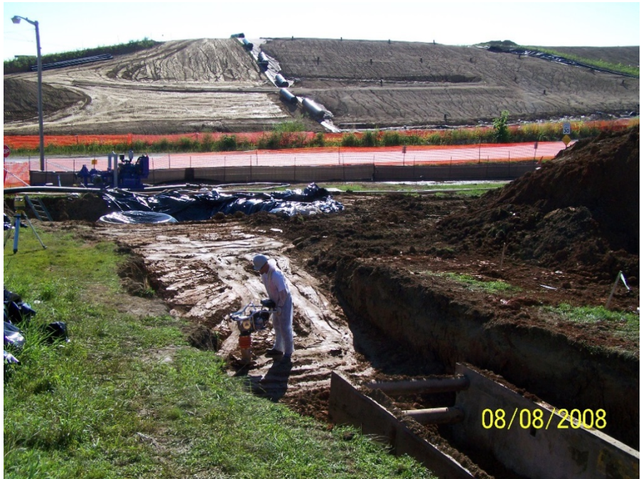
Photo No. 34: AOI 21-2 – Compaction of backfill around storm sewer, facing east. August 2008.
