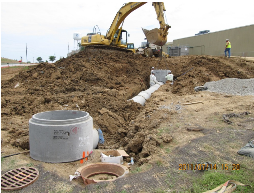
Photo No. 49: AOI 21-2 – Installation of storm sewer piping for parking lot drainage, facing southwest. July 2011.
