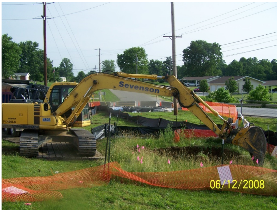
Photo No. 26: AOI 21-1 – Excavation of \geq 50 mg/kg PCBs material, facing northeast. June 2008.
