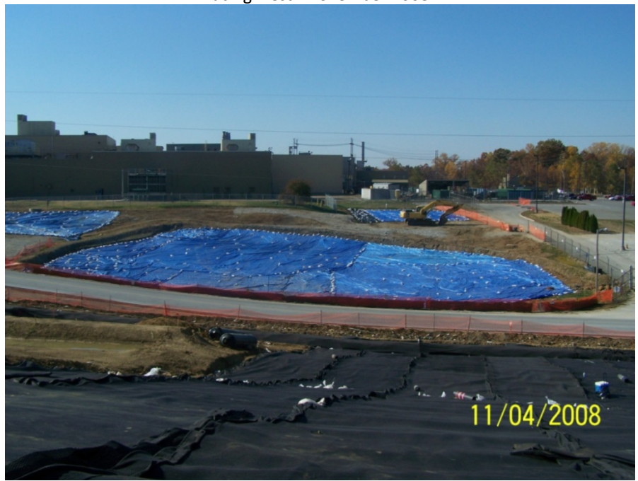
Photo No. 43: AOI 21-2 – Temporary cover, pending temporary soil cover placement, facing west. November 2008.
