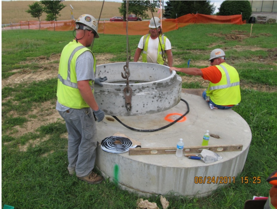
Photo No. 48: AOI 21-2 – Raising of manhole to accommodate final parking lot elevation, facing southeast. June 2011.
