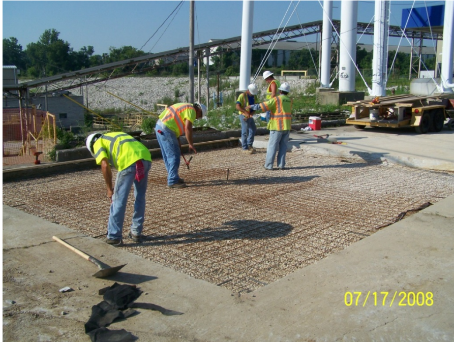
Photo No. 20: AOI 18 – Placement of wire mesh prior to concrete pour, facing southwest. July 2008.
