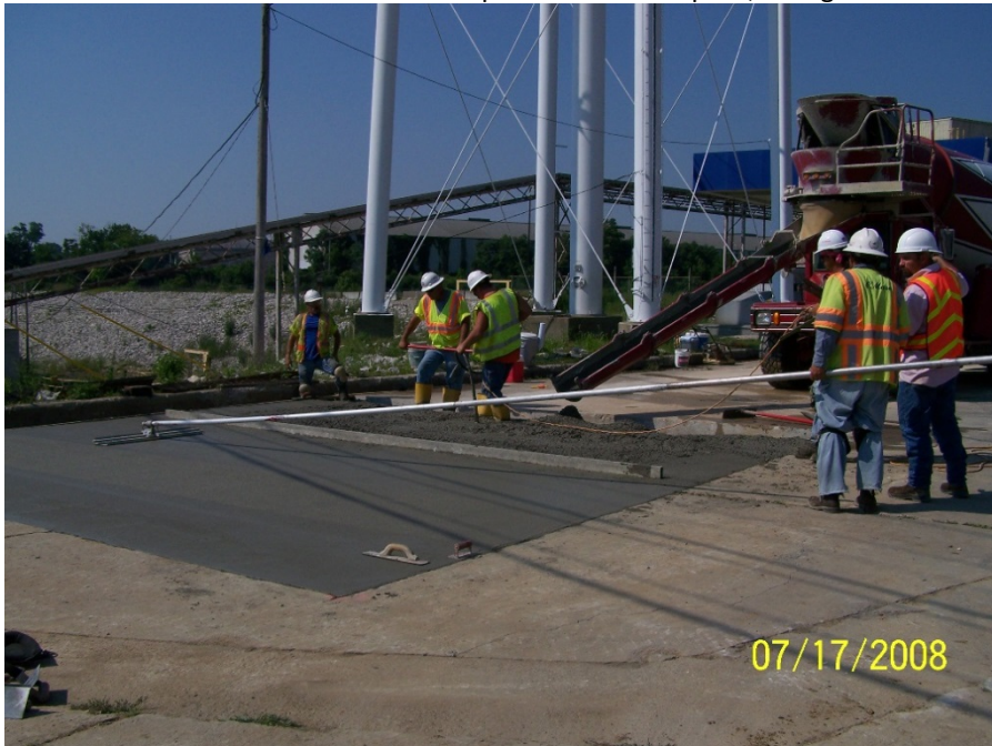
Photo No. 21: AOI 18 – Installation of concrete pad (air intrusion, leveling, and smoothing), facing southwest. July 2008.
