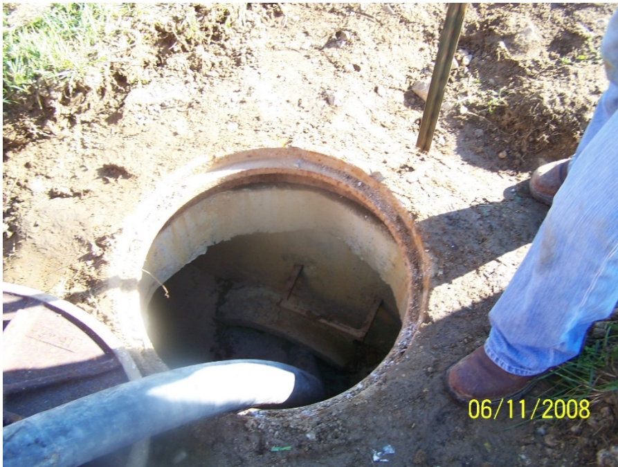
Photo No. 4: MH-ST-43 – Introduction of flowable fill into pipes, facing down. June 2008.
