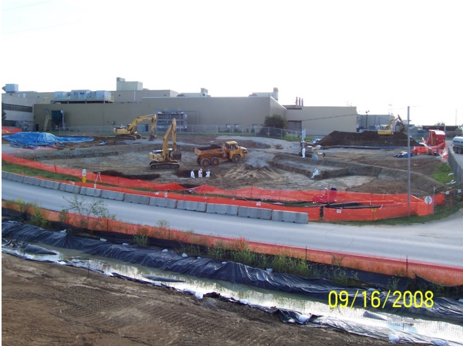
Photo No. 38: AOI 21-2 – Excavation of \geq 50 mg/kg PCB material lens, facing southwest. September 2008.
