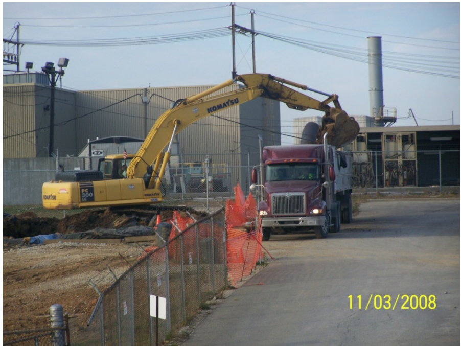
Photo No. 42: AOI 21-2 – Loading \geq 50 mg/kg PCB material for disposal at Heritage Landfill in Roachdale, Indiana, facing west. November 2008.
