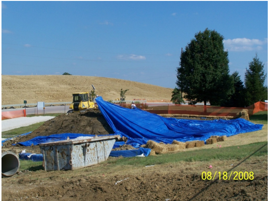
Photo No. 36: AOI 21-2 – Placement of temporary cover for <50 mg/kg PCB material stockpile, facing southwest. August 2008.
