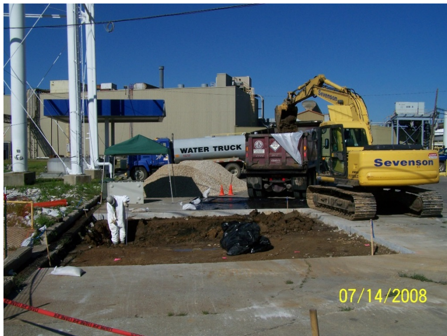
Photo No. 17: AOI 18 - Excavation of \geq 50 mg/kg PCB material, facing west. July 2008.
