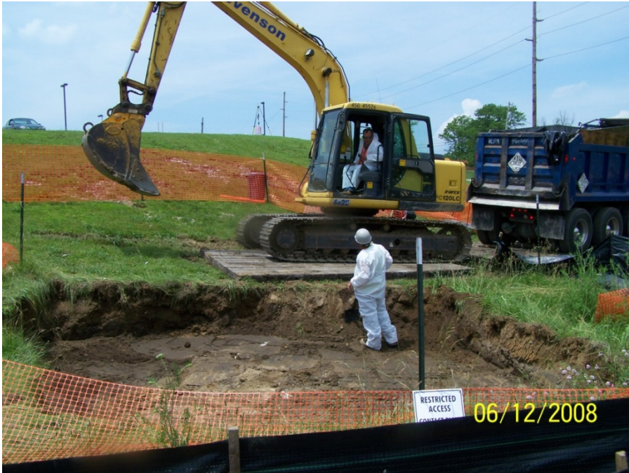
Photo No. 28: AOI 21-1 – Excavation of \geq 50 mg/kg PCBs material, facing west. June 2008.
