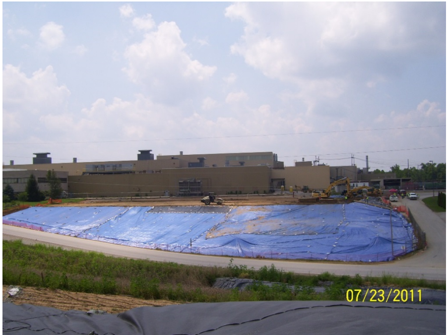
Photo No. 52: AOI 21-2 – Erosion protection of clay barrier layer, facing west. July 2011.
