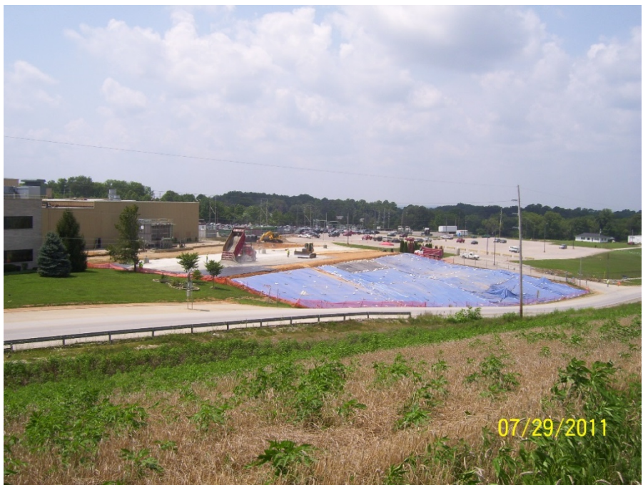
Photo No. 53: AOI 21-2 – Placement of gravel base for parking lot, facing northwest. July 2011.
