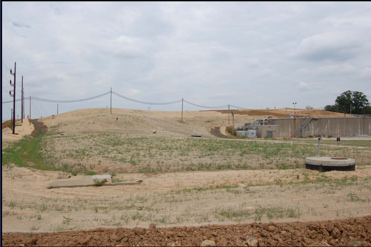
Completed cover area off of GM Drive. Small amount of grading seeding remains.
