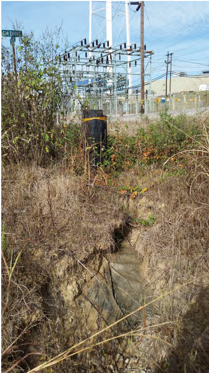
Photo 10: EV6 erosion rut outside cap limit
