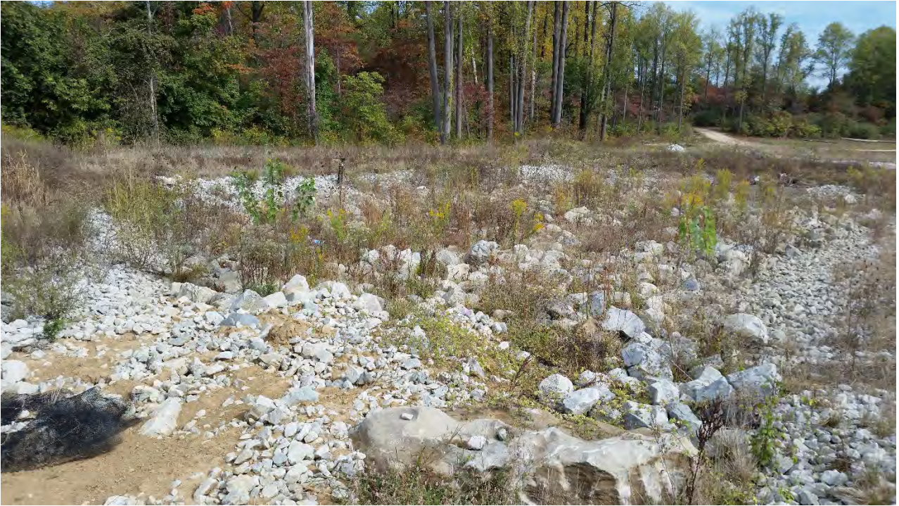
Photo 26: ES9 rip rap erosion at storm drain into detention basin #2 facing west
