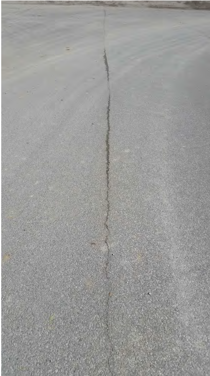
Photo 31: EA2 facing east, cracks in asphalt west of Parcel 205
