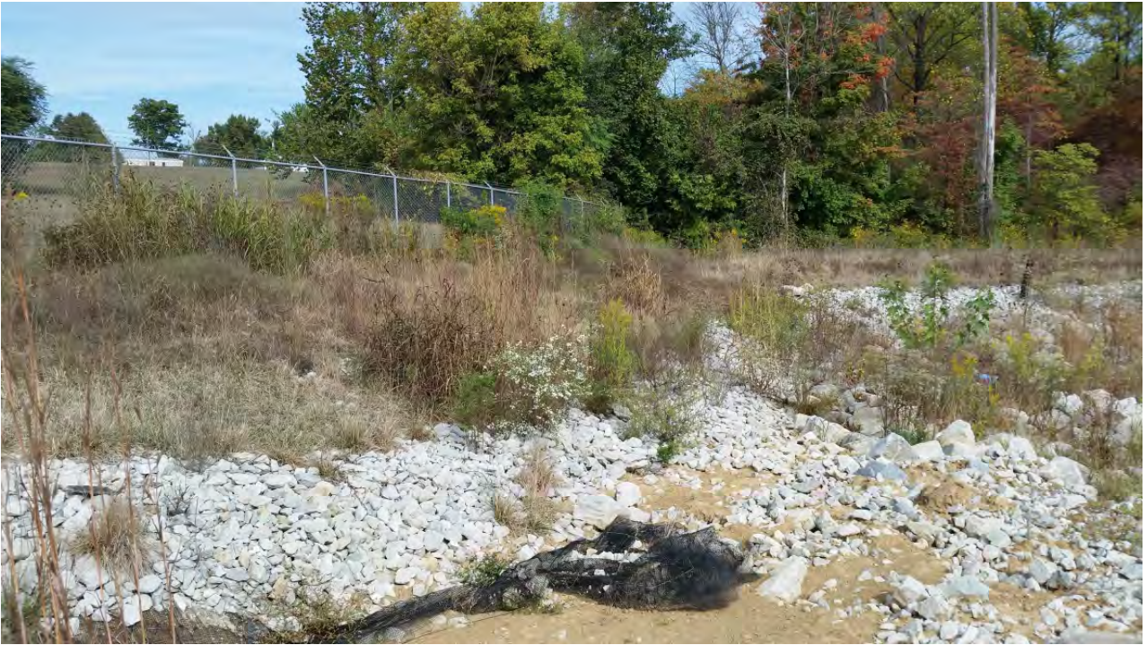
Photo 24: ES6 drainage swale facing west, channel erosion.
