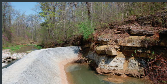
SPRING 018 CONTAINMENT BERM
