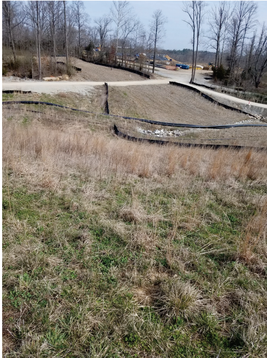
Photo 11: EV4 East Plant Area Cover looking northeast toward ES11 East Plant Area Cover.
