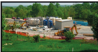
New Waste Water Treatment Facility
