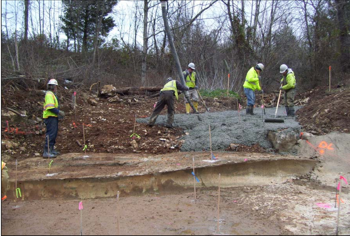
PHOTO No. 19: BEGINNING OF CONCRETE POUR WHERE TRIBUTARY 2 DISCHARGES INTO BAILEY'S BRANCH. DEC. 2012
