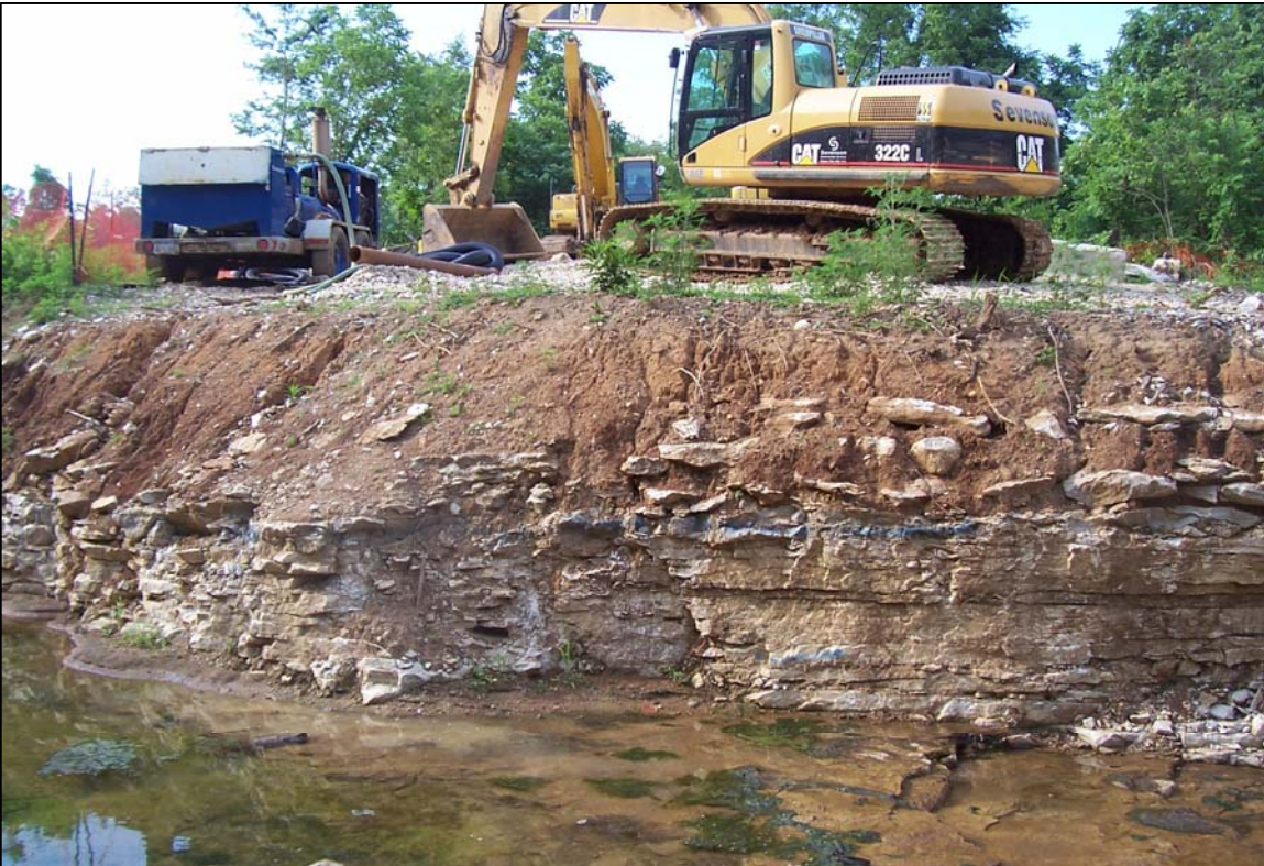
PHOTO No. 13: TYPICAL EXPOSED CREEK SIDEWALL FOLLOWING EXCAVATION ALONG TRIBUTARY 3 AND BAILEY'S BRANCH CREEK ON PARCEL 216, PRIOR TO SHOTCRETE APPLICATION. JULY, 2005
