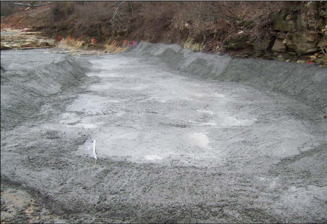
PHOTO No. 28: COMPLETED BASEFILL CONCRETE FOR THE POND CONSTRUCTION NEAR FORMER SWALLET 7, LOOKING UPSTREAM, DEC. 2012
