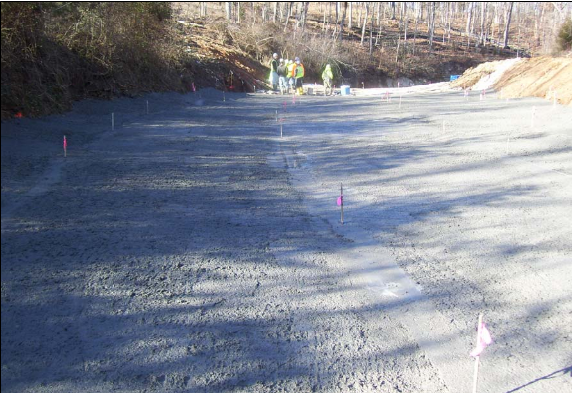
PHOTO No. 23: CONCRETE WORK LOOKING FROM CONFLUENCE TOWARD SWALLET 7 ALONG CENTERLINE DEC. 2012
