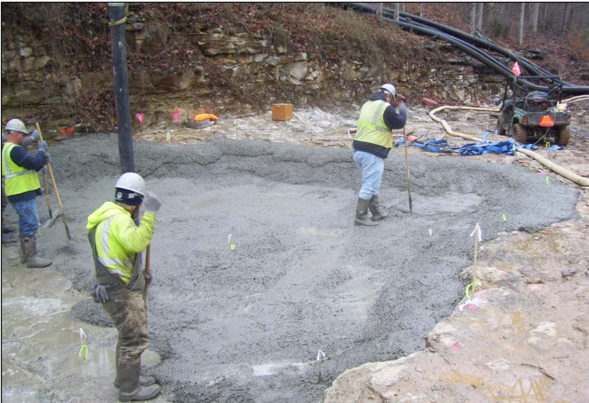
PHOTO No. 26: POURING CONCRETE FOR THE POND CONSTRUCTION NEAR FORMER SWALLET 7. DEC. 2012
