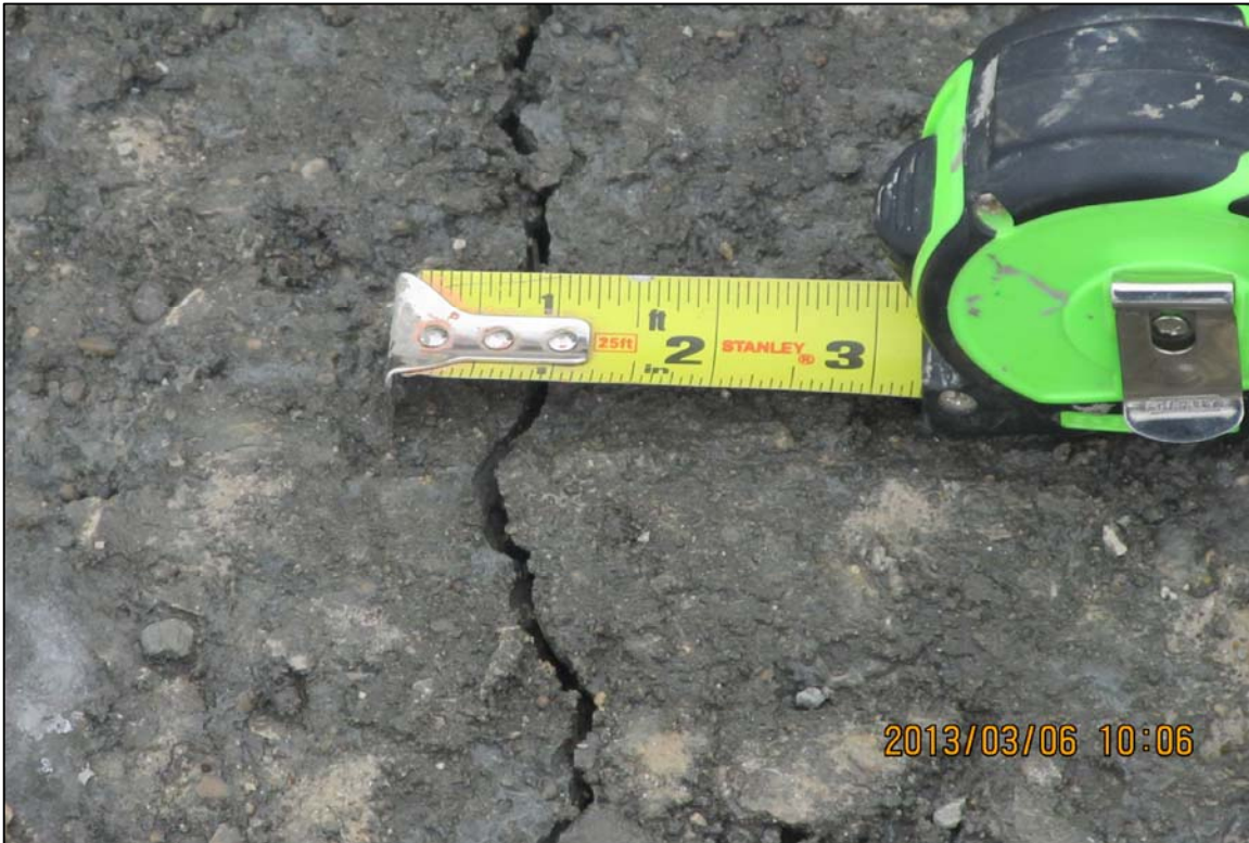
PHOTO No. 40: TYPICAL CRACK PRIOR TO REPAIR. MAR. 2013
