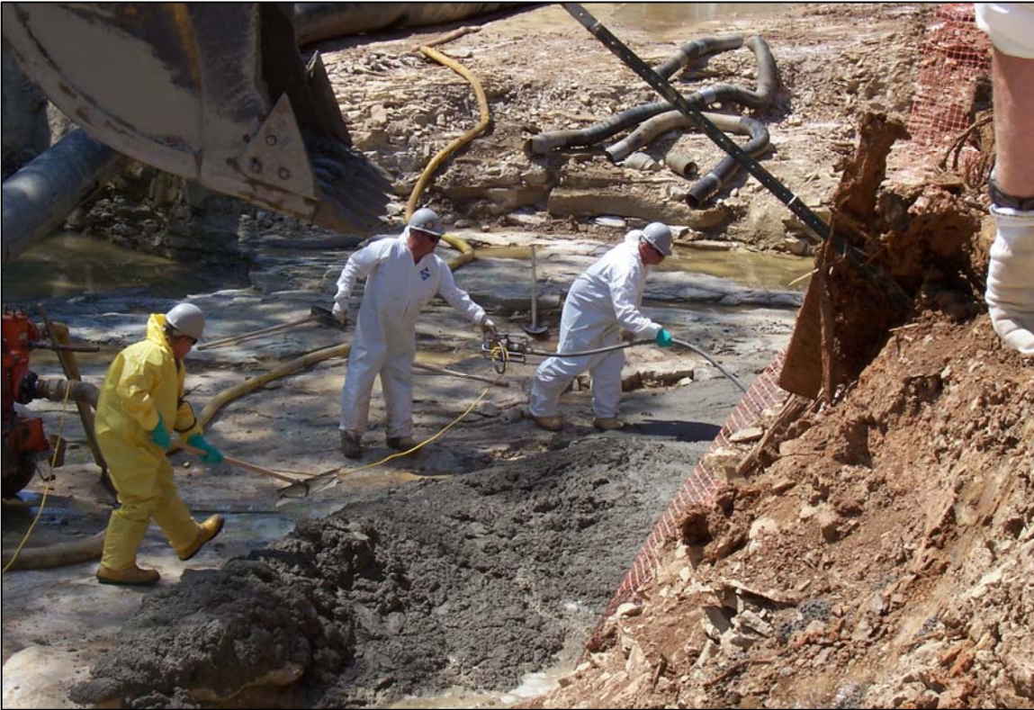
PHOTO No. 12: SIMULTANEOUS WATER PUMPING AND CONCRETE FILLING AT SWALLETS 2 AND 3. MAY, 2005
