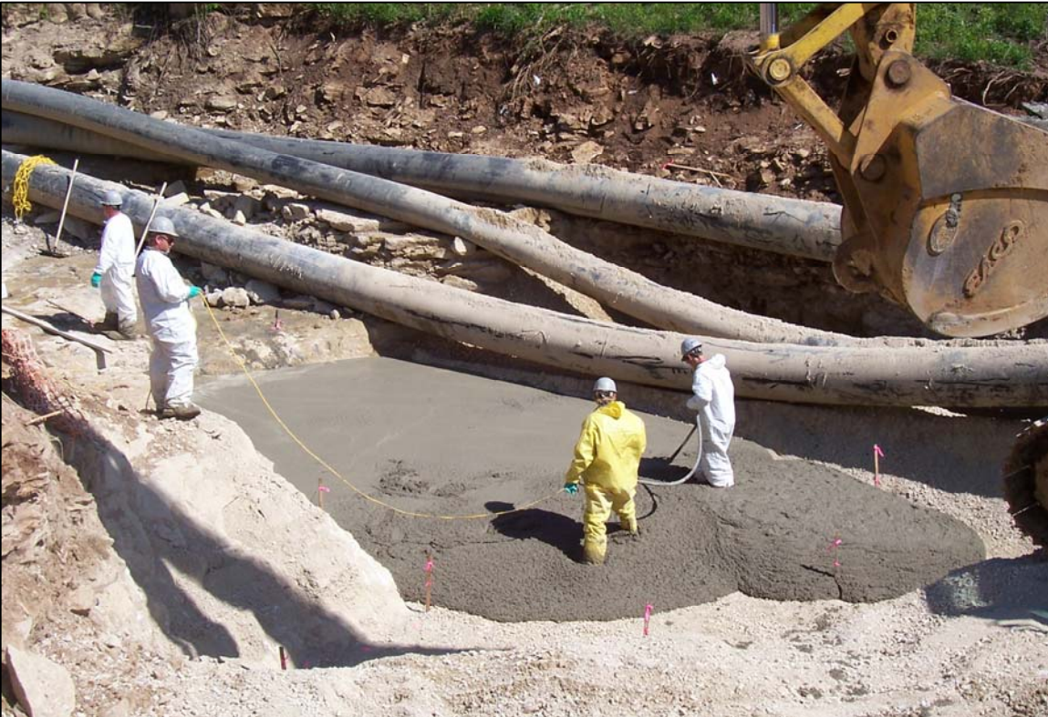
PHOTO No. 10: CONCRETE FILLING OF SWALLETS 1A AND 1B BEDROCK TRENCH. MAY. 2005
