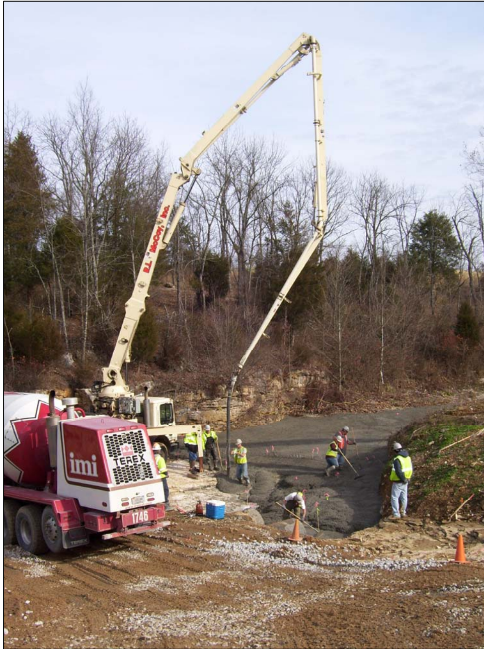
PHOTO No. 18: PUMP TRUCK POURING BASEFILL CONCRETE OF SEALING LAYER UPSTREAM OF TRIBUTARY 3, DEC. 2012
