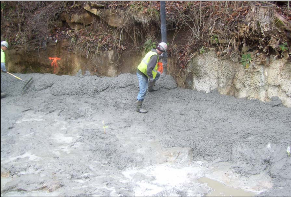
PHOTO No. 27: POURING CONCRETE ALONG THE CREEK SIDEWALL OVER PREVIOUSLY SHOTCRETE WITHIN POND NEAR FORMER SWALLET 7, DEC. 2012
