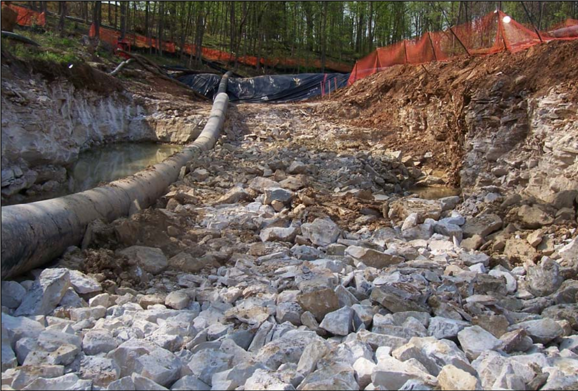
PHOTO No. 9: BROKEN OUT ROCK NEAR SWALLETS 2 AND 3 TO BE HAULED OUT. APR. 2005
