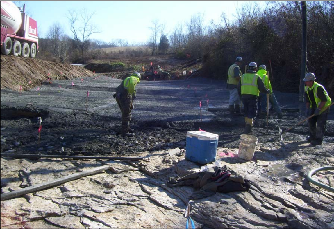
PHOTO No. 22: CONCRETE WORK LOOKING FROM SWALLET 7 AREA UPSTREAM TOWARD TRIBUTARY 3 CONFLUENCE, DEC. 2012
