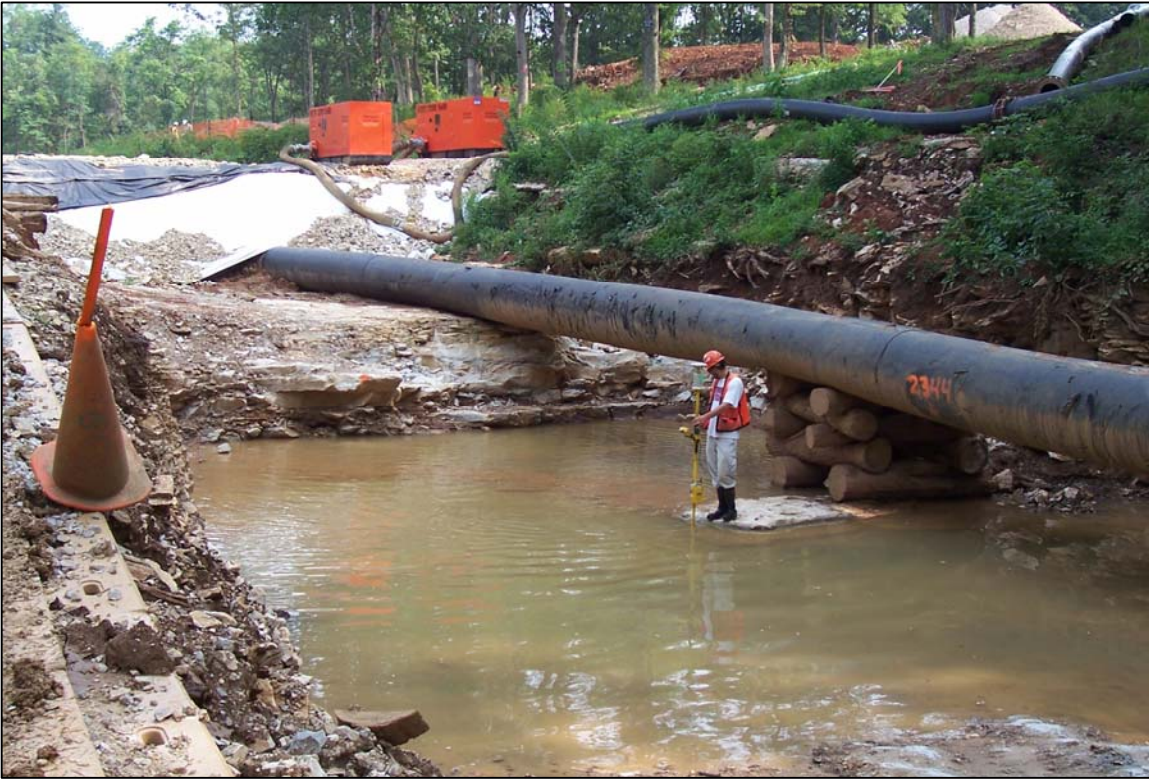
PHOTO No. 16: CRA SURVEYOR LOCATING THE CONCRETE POURED NEAR SWALLET 7, ADJACENT TO THE CREEK BY-PASS PIPING, AUG. 2005
