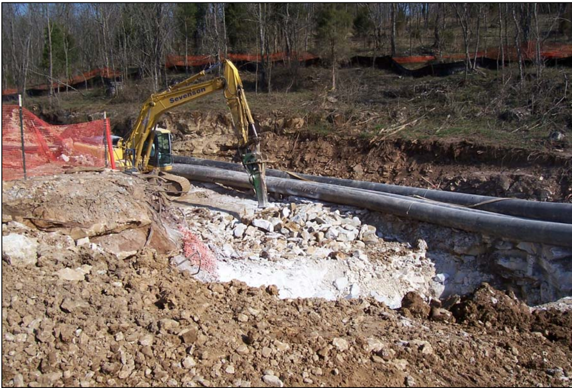
PHOTO No. 7: BEDROCK FRACTURES BEING BROKEN-OUT IMMEDIATELY DOWNSTREAM OF SWALLETS 1A AND 1B. APR. 2005
