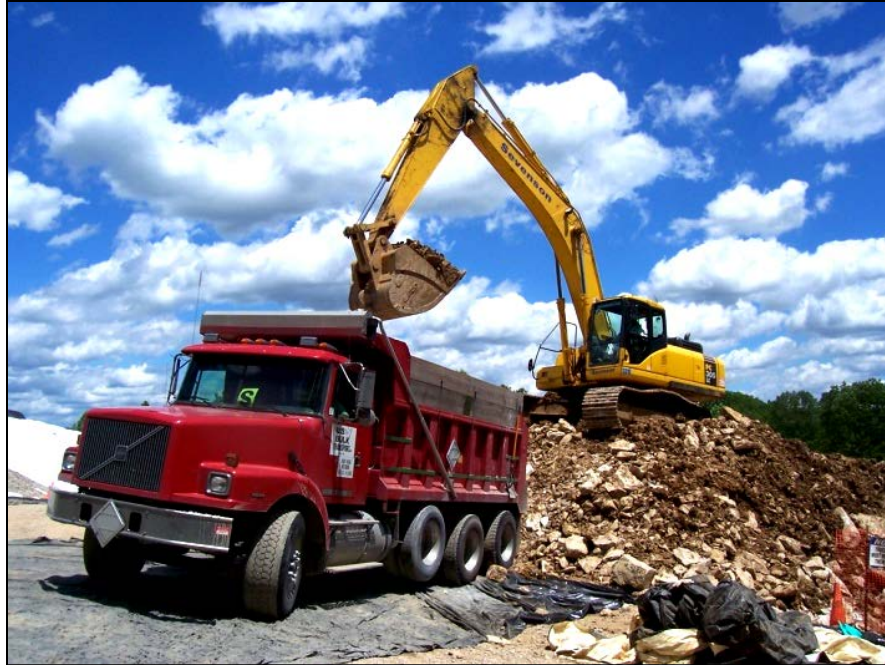
Photo No.3: Parcel 216 - Loading Excavated Creek Material to be used for Grading Fill (Facing Northeast). June 2005
