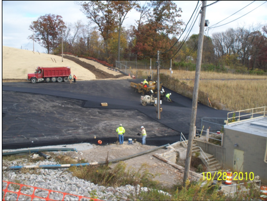
Photo No.79: AOI-8 – Gravel Base for Asphalt Cover System (Facing Northeast). October 2010
