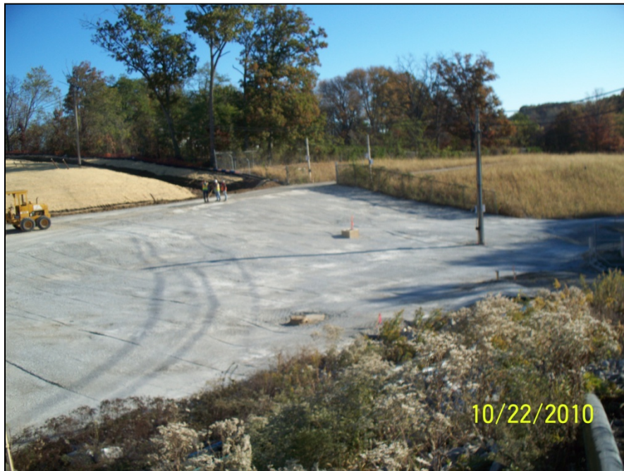
Photo No.78: AOI-8 – Gravel Base for Asphalt Cover System (Facing Northeast). October 2010
