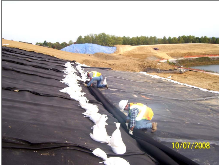
Photo No.37: AOI-4 - Installation of perforated drainage pipe and geocomposite material (Facing North). October 2008
