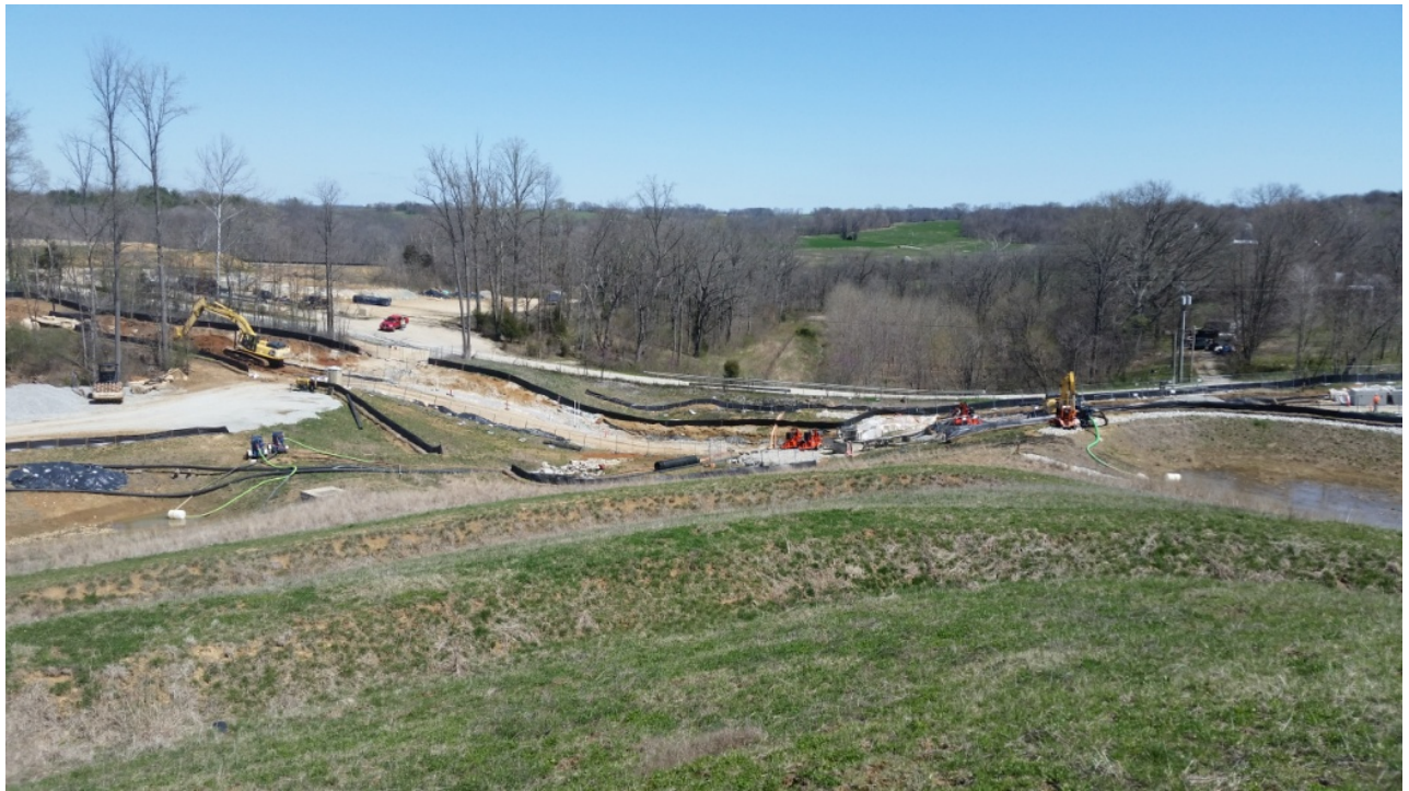
Photo 3: Looking Northeast along EV4 East Plant Area Cover toward ES7, ES8, ES10, and ES11
