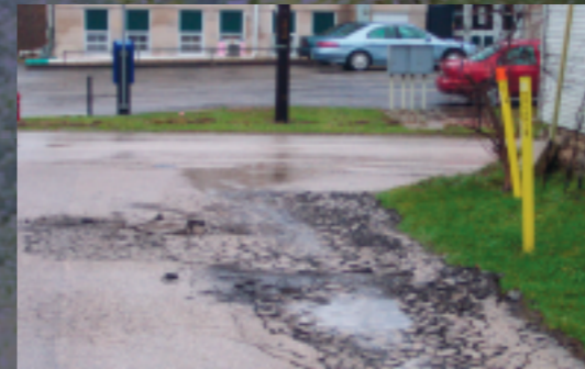
Damaged Road Shoulder
