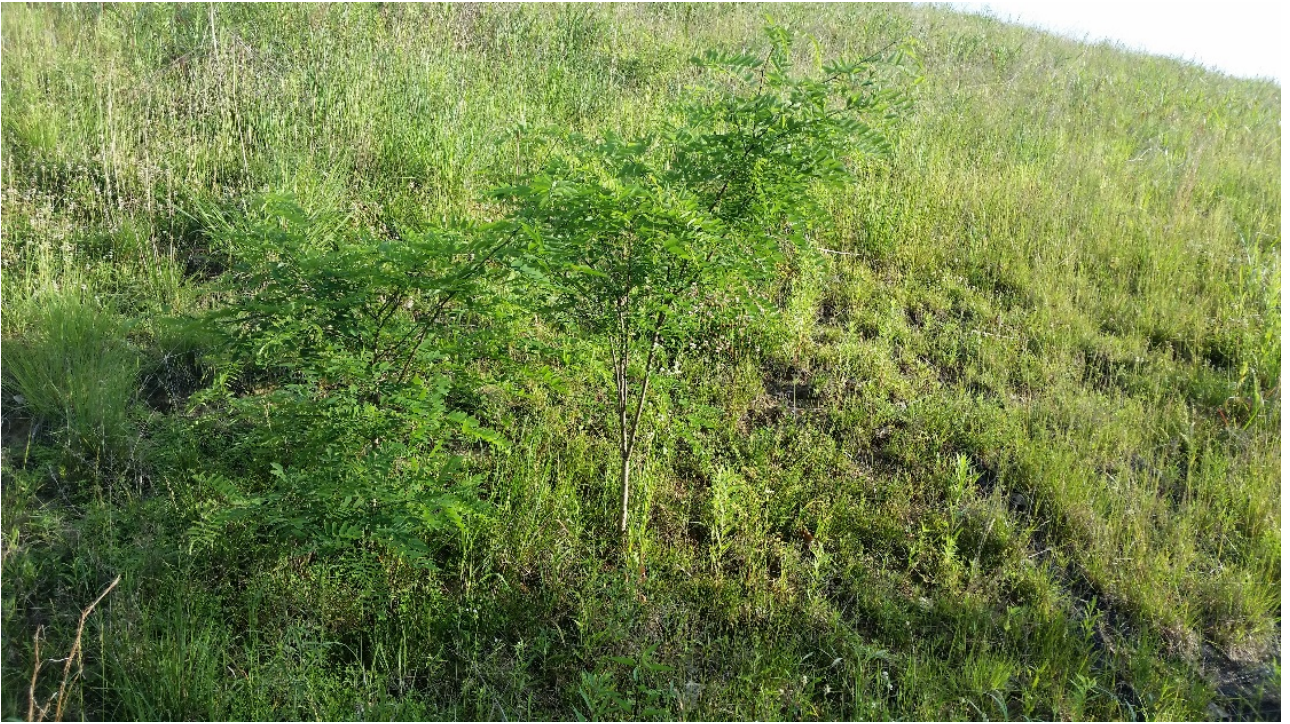
Photo 12: EV9 East Plant Area cover facing south (removed tree growth at time of inspection)
