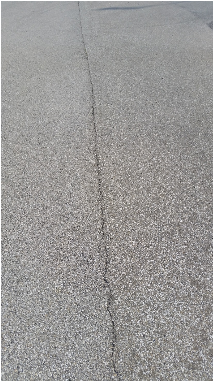
Photo 24: EA2 crack near WWTP aeration basin facing north
