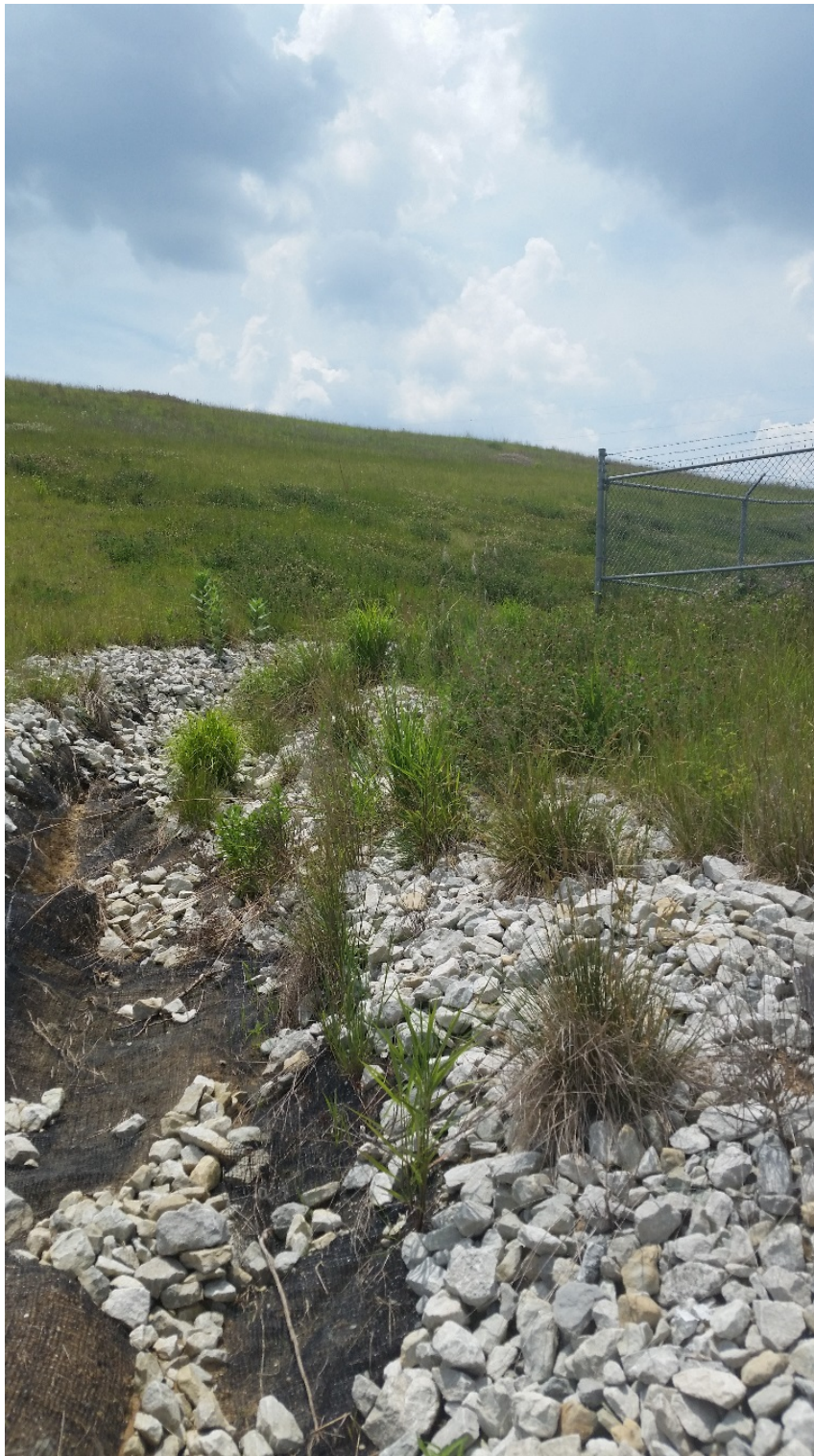
Photo 20: ES6 drainage swale facing southwest, channel erosion.
