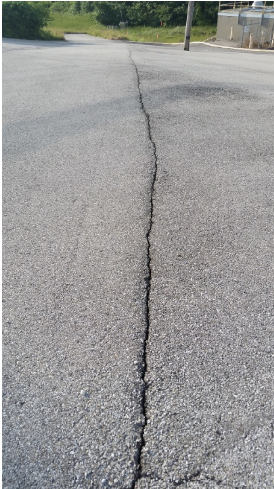
Photo 25: EA2 facing east, cracks in asphalt west of Parcel 205
