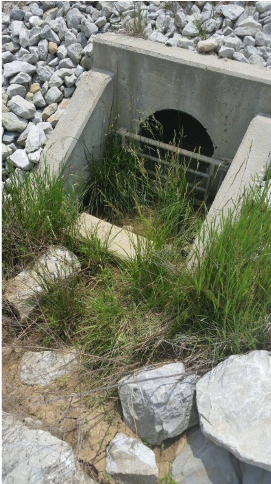
Photo 21: EV9 rip rap erosion at storm drain into detention basin #2 facing west
