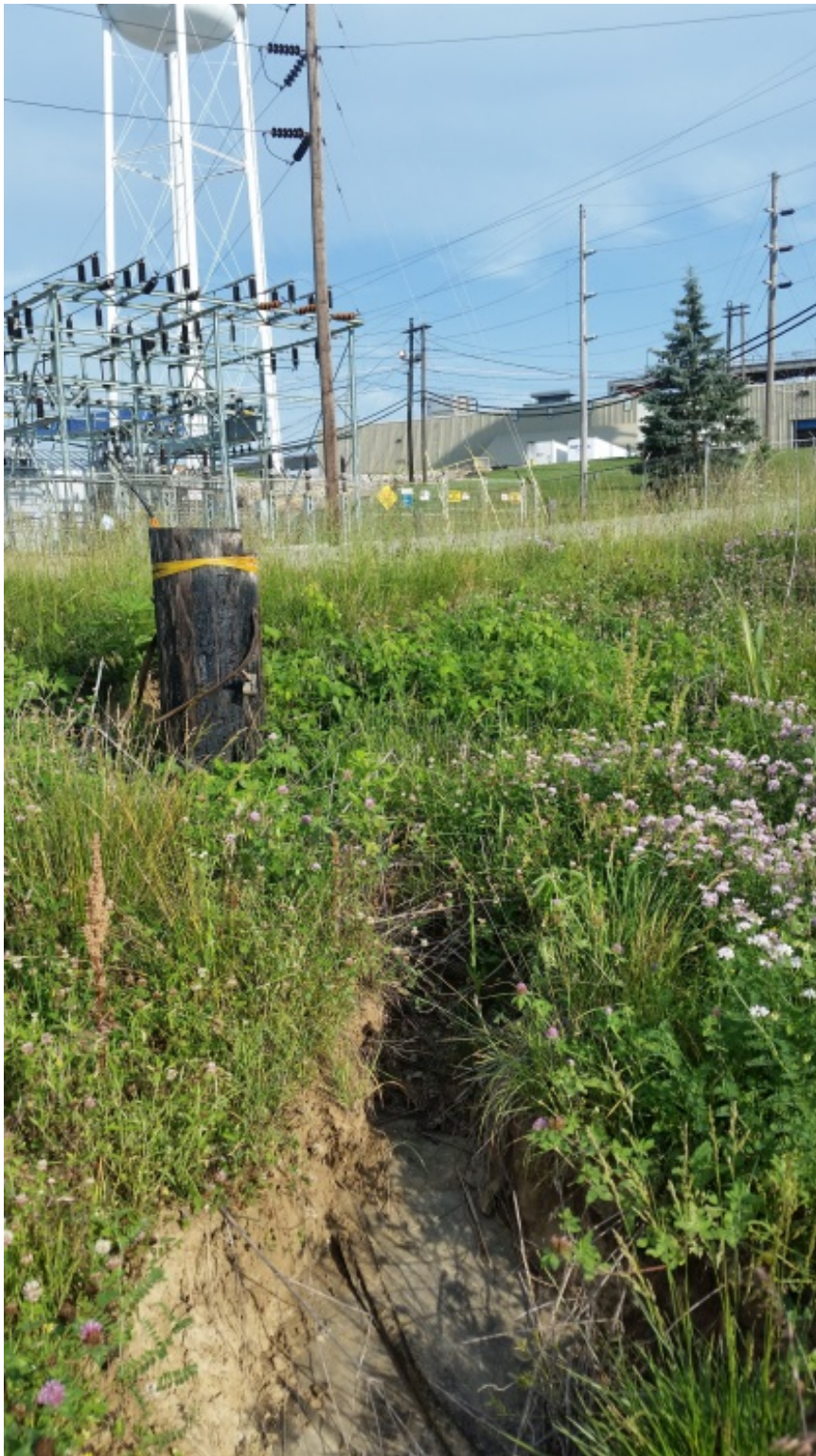
Photo 9: EV6 erosion rut outside cap limit
