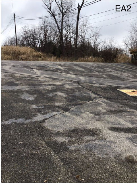
Photo 3 Looking north, example of asphalt cracks to be filled
